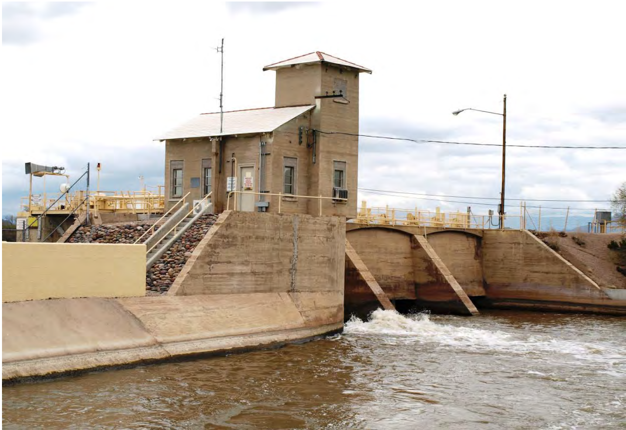
Photo 6. Granite Reef Diversion Dam south gate structure and South Canal turnout looking northeast.
