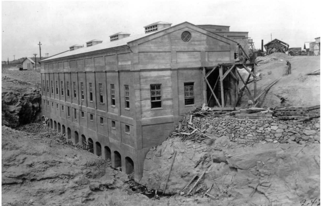
Historic Photo 7. Crosscut Hydro Plant under construction, 1913. Photo courtesy of the SRP.
