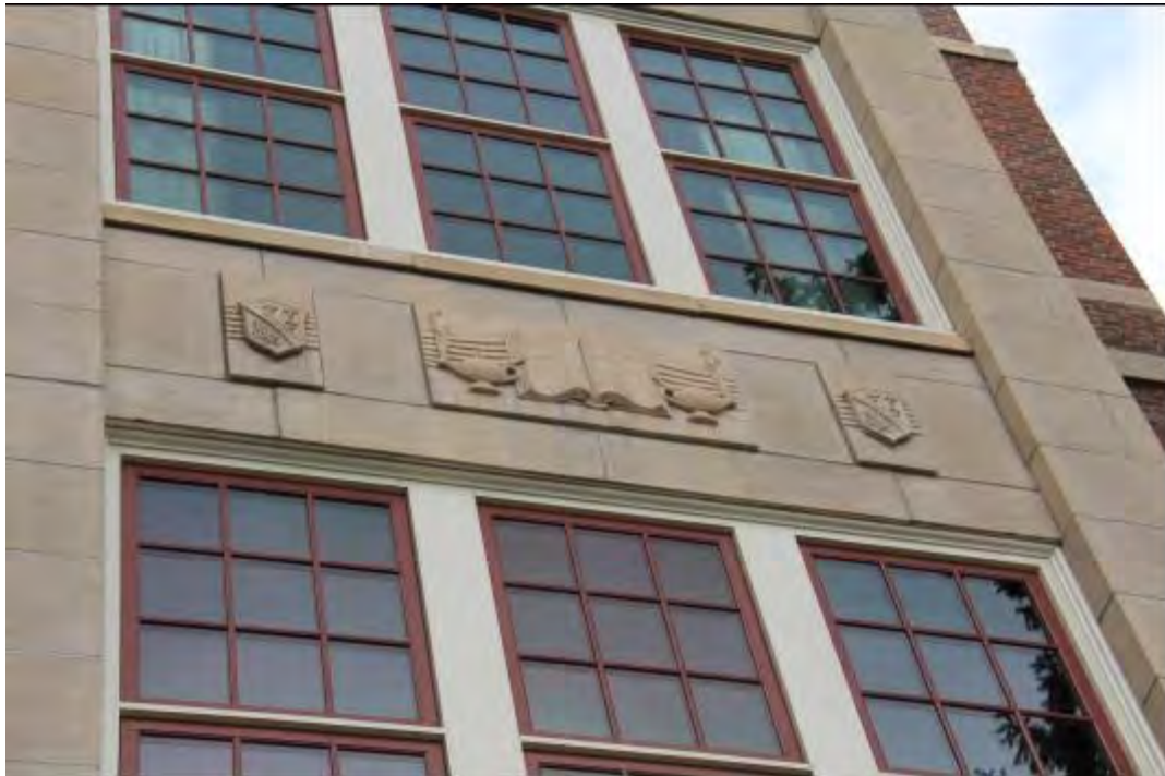
0010 Detail photo of cultured stone panels and raised inserts above the front entry. View to north.
