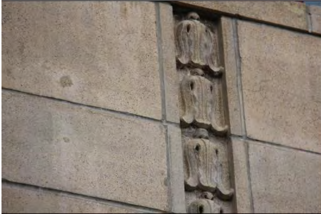
0011 Detail photo of cultured stone panels and lotiforms that are distributed around the building.
