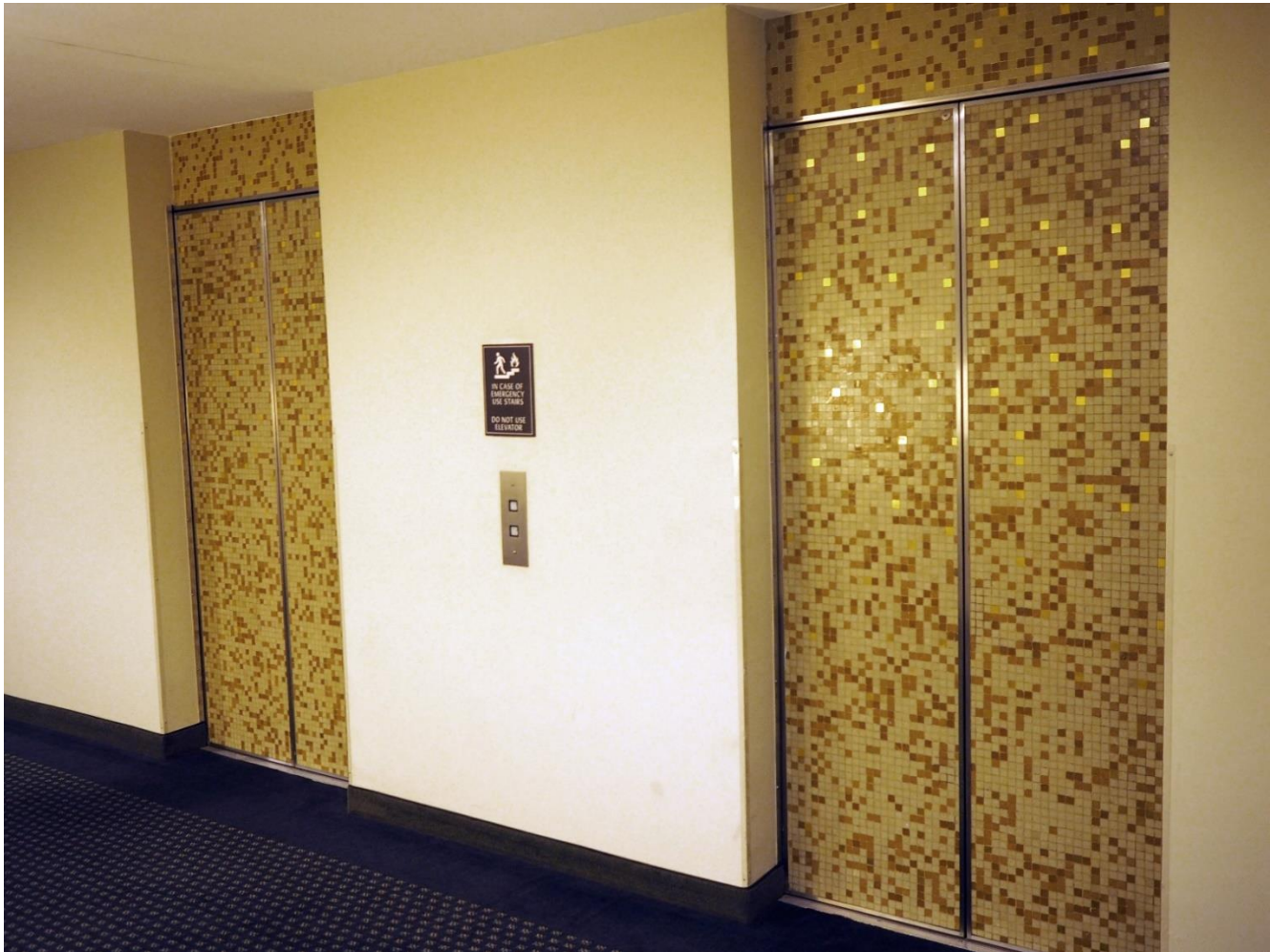
Photo 14. Current photograph of a typical set of elevator doors on a residential floor.
