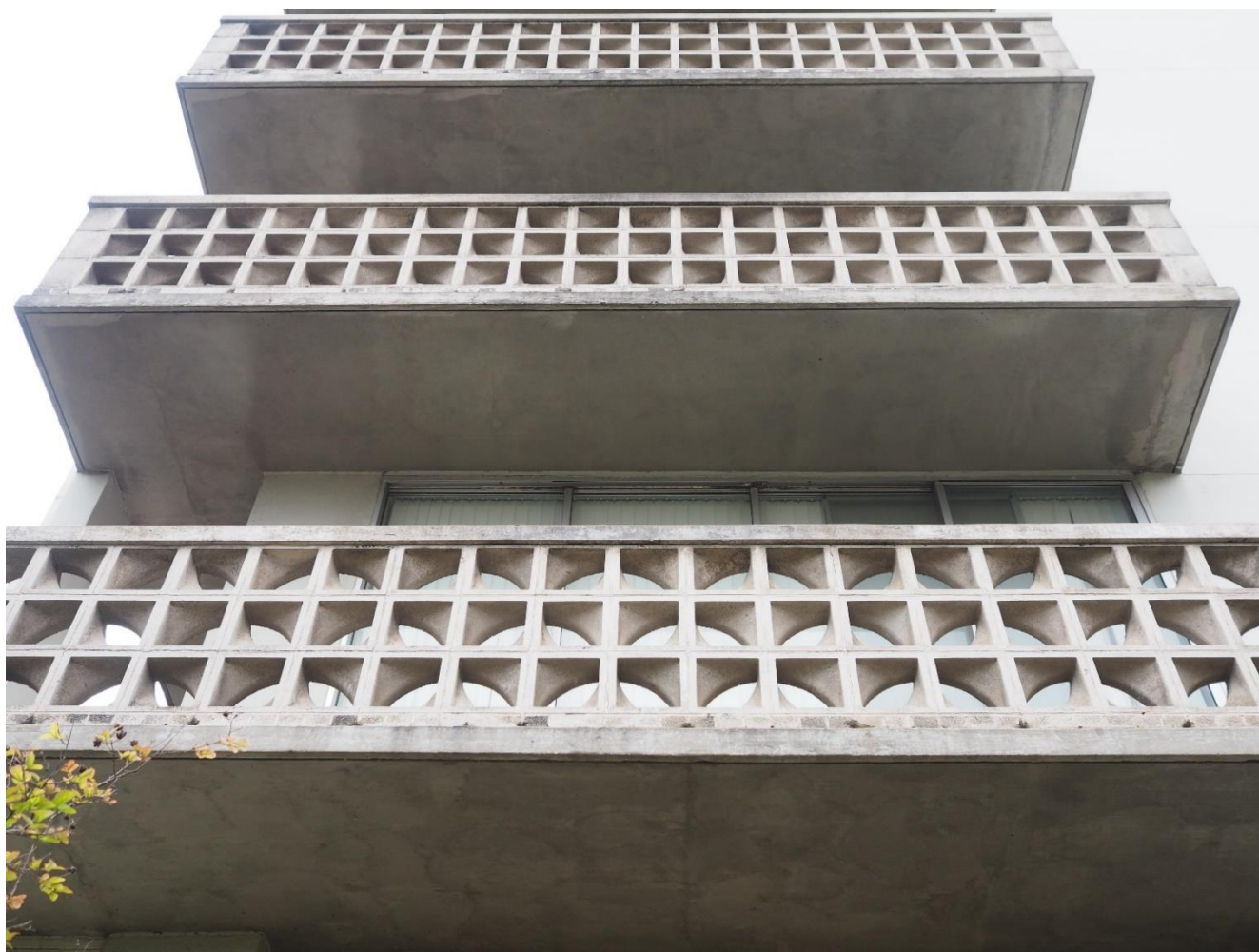
Photo 5. Current photograph of a typical balcony on the north corner of the building.
