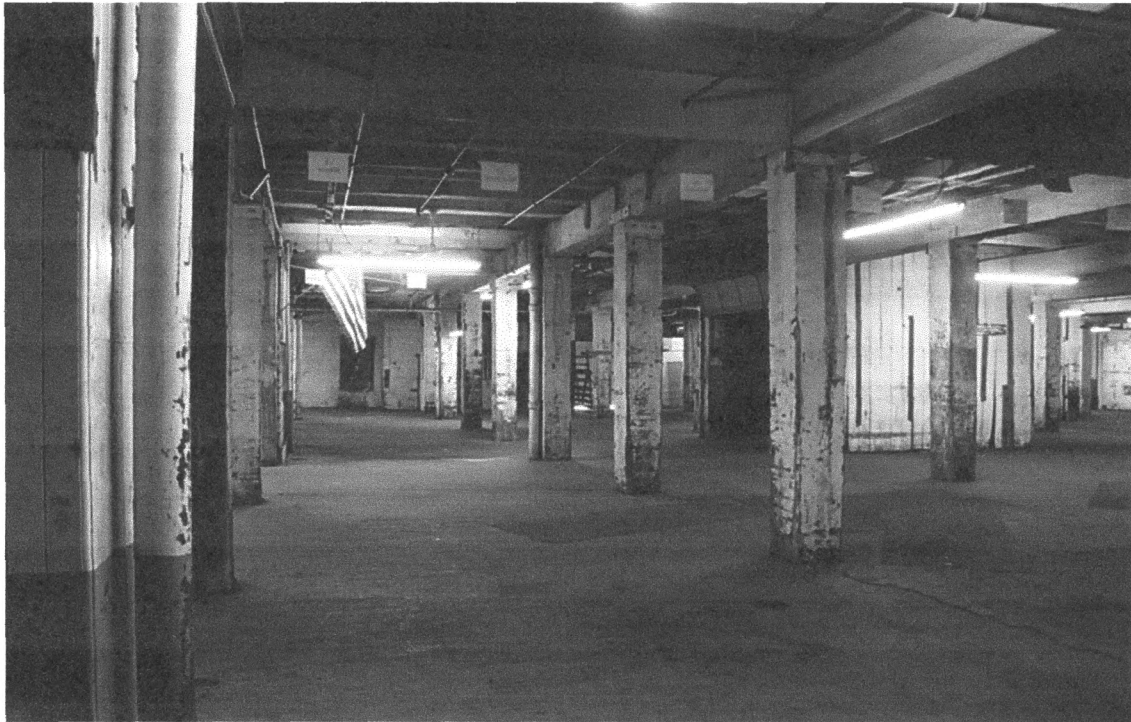
Figure 12 The heavy timbers of the interior structure are encased in beadboard siding and painted on the first floor. Here the view was taken from the northeast corner of the building. Mike Whye photograph, 2007.
