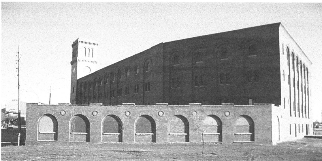
Figure 11 The single-story appendage to the main building was intended to serve as office and showroom space. The building plans mark the interior space behind the far left arch (formerly a window) as the “Directors” room and include a fireplace (nonextant). The third arch from the right was a blind arch from the start and concealed a room-size vault inside. The two arches to its right likely had window glass only in the top arch spaces, as men’s and women’s restrooms were located inside. This view looks southeast at the appendage and, behind it, the north side and northwest sides of the warehouse building. Note the slight angle change of the wall four bays from the left corner. Mike Whye photograph, 2007.
