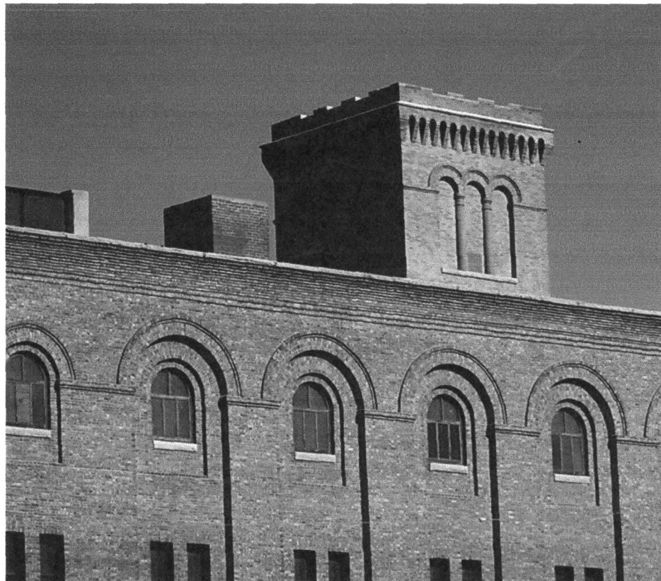
Figure 6 Rising behind the fourth floor windows of the south elevation, the six-story crenellated tower was intended to serve multiple purposes for the Simmons Hardware Company: hide a water tank, demarcate the main entrance to the massive building, provide the public and workers with the time of day, and perhaps, most importantly, create a landmark and suggest the importance of the Simmons Hardware Company, much like the landmark clock tower of the U.S. Post Office (later City Hall) suggested the importance of the federal government. Mike Whye photograph, 2007.
