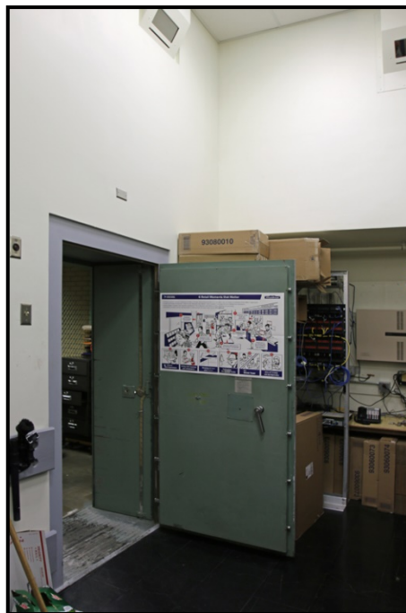
Photograph 12. Vault security door in the post office workroom, facing southeast. Note the observation portals for the former workroom catwalk along the ceiling.
