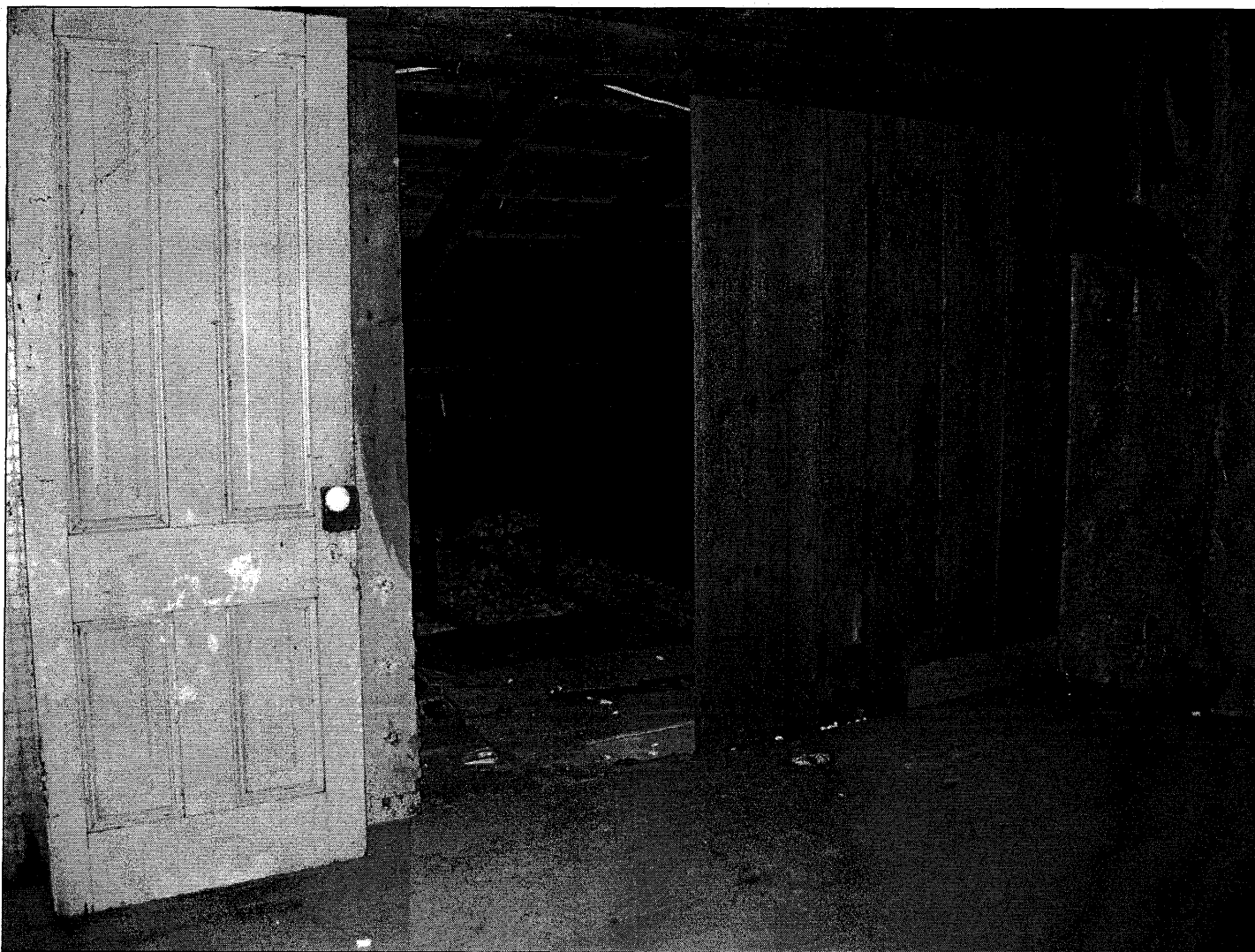
Photo 21 of 22. Attic, west bedroom, south wall, looking south/southwest. Door appears to be only remaining original or early door in the house. Planks form structural wall extending from sill to top plat (visible along top of photo). Sloping roof beyond plank wall encompasses "saltbox" section along south elevation that includes kitchen, bathroom and bedroom on first floor.
