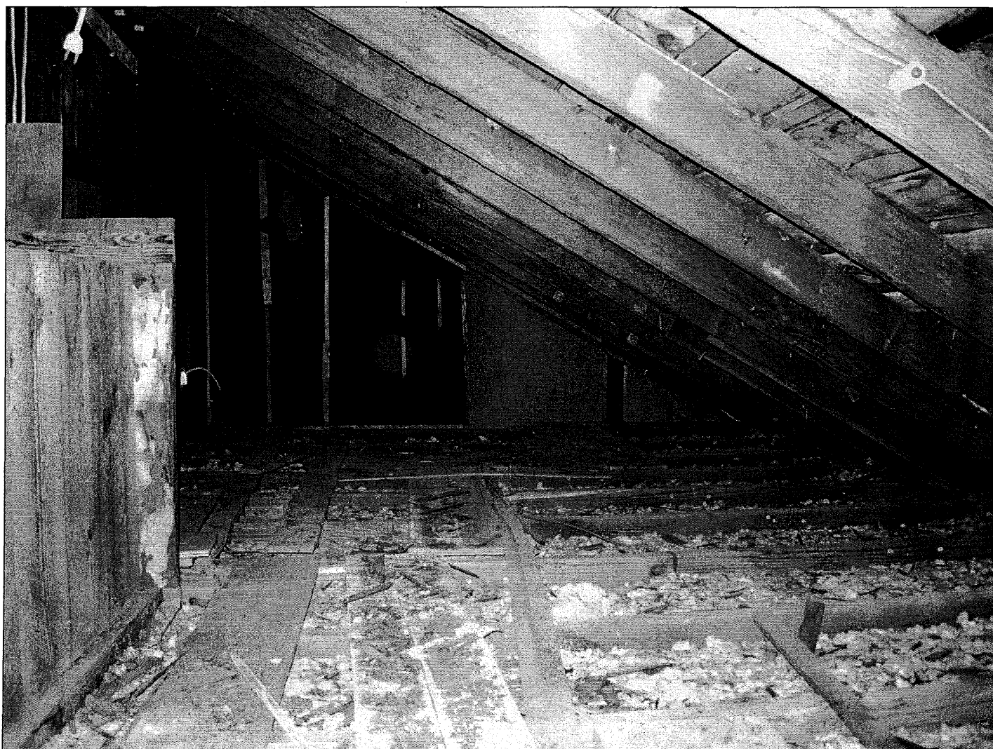
Photo 22 of 22. View of framing inside south wing roof portion of house, looking east. This section is attached to southern plank wall (at left), and consists of stud wall construction with horizontal board sheathing.
