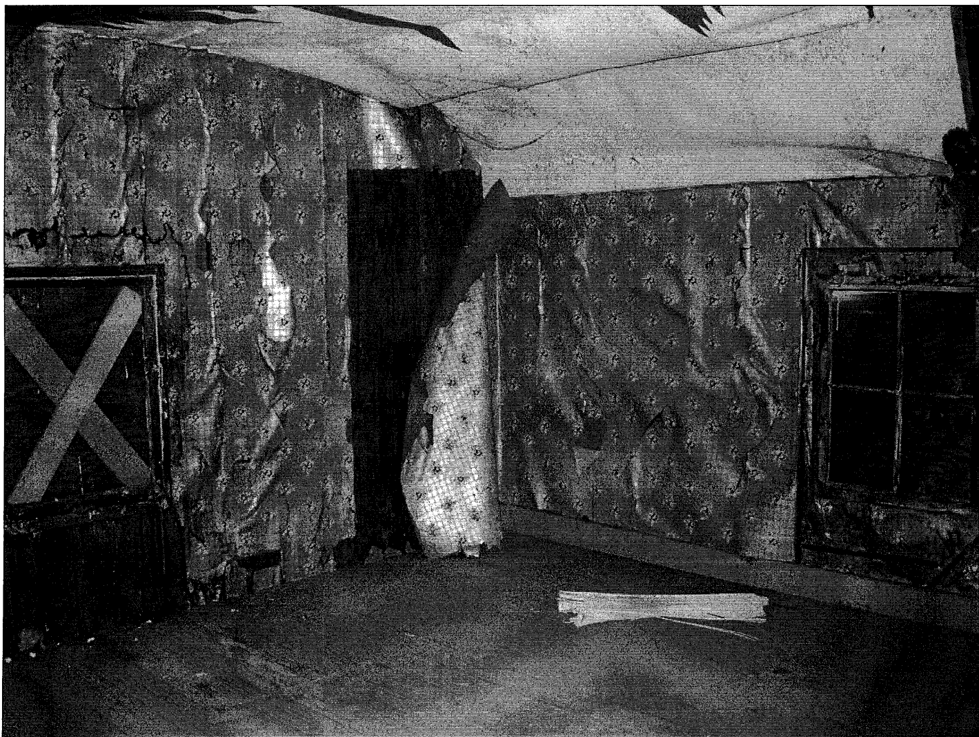
Photo 20 of 22. Attic, west bedroom. Barely visible in left lower portion of photo is patch in flooring marking possible location of original stair. View looking northwest.
