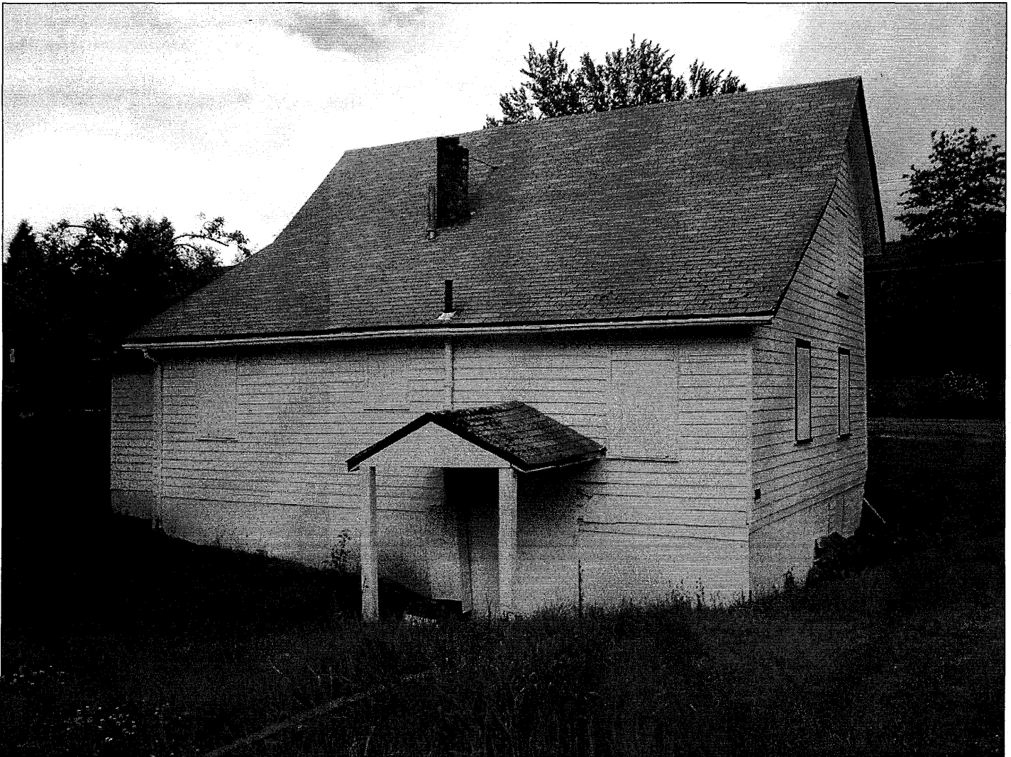
Photo 4 of 22. South (rear) elevation. Note dip in topography and recent fill at right of photograph.
