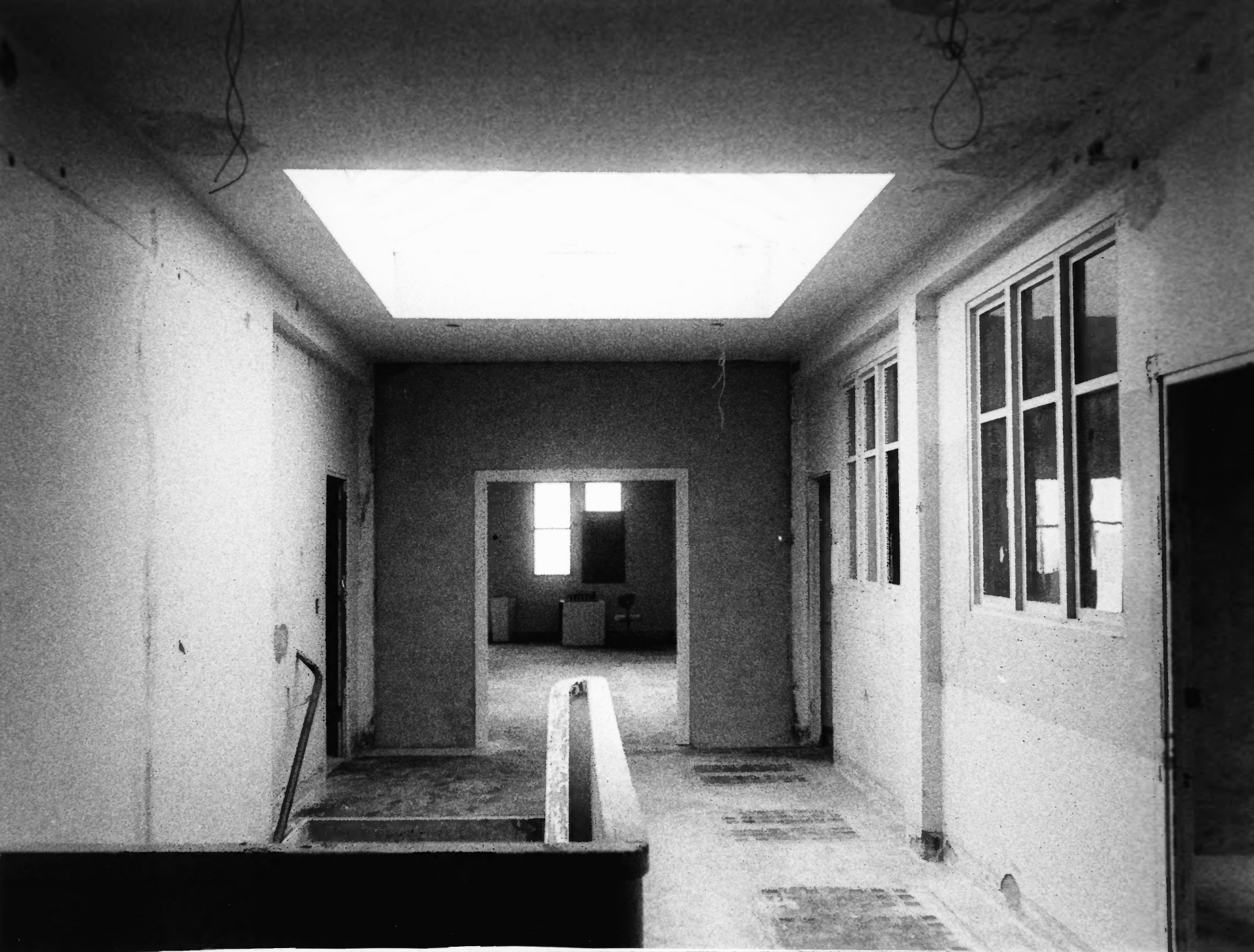
Upstairs corridor (toward classroom). Skylight, interior windows, and sidewalk lights visible. (Photo taken in natural light.) (1980)
