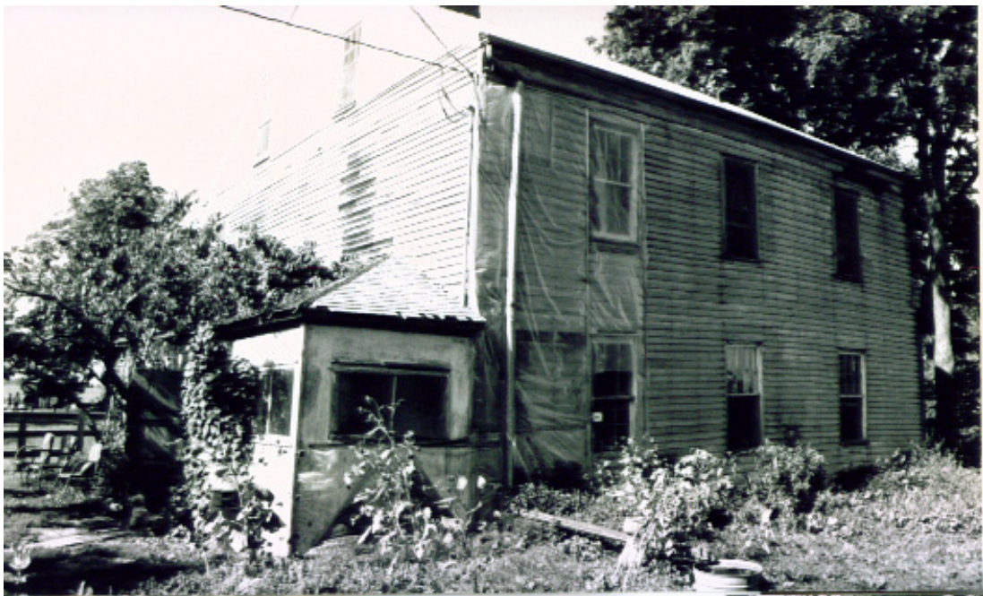
Figure 11. Top. The northern and western sides of the inn. Bottom. The northern and eastern sides with later porch addition. Photos 1992 by author.
