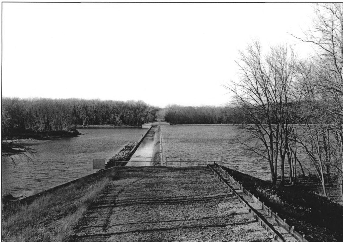
PHOTO 4. Detail of Stationary Section of Dam, Concrete-Covered Ogee Spillway Submersible Earth- and Sand-filled Dike, Which is the Middle of the Three Dikes Which Make Up the Stationary Portion of the Dam.
