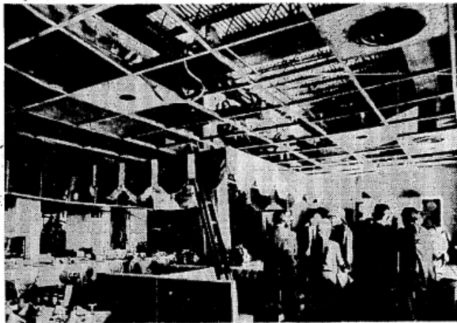
CEILING PANELS in the dining room of the Governor House Motel were shattered and fell when a structural failure caused collapse of five floors and roof of the building Friday. Officials inspect the damage in the area.
