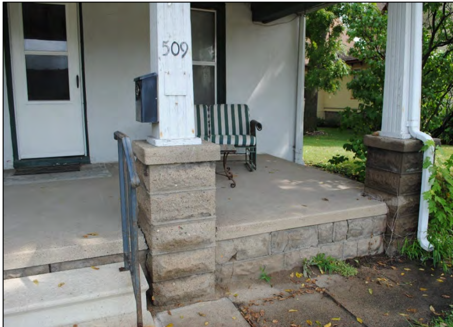
Figure 20. Detail of the front porch posts and piers/ foundation looking NE. Photograph taken 08-07-2018 by Tallgrass.
