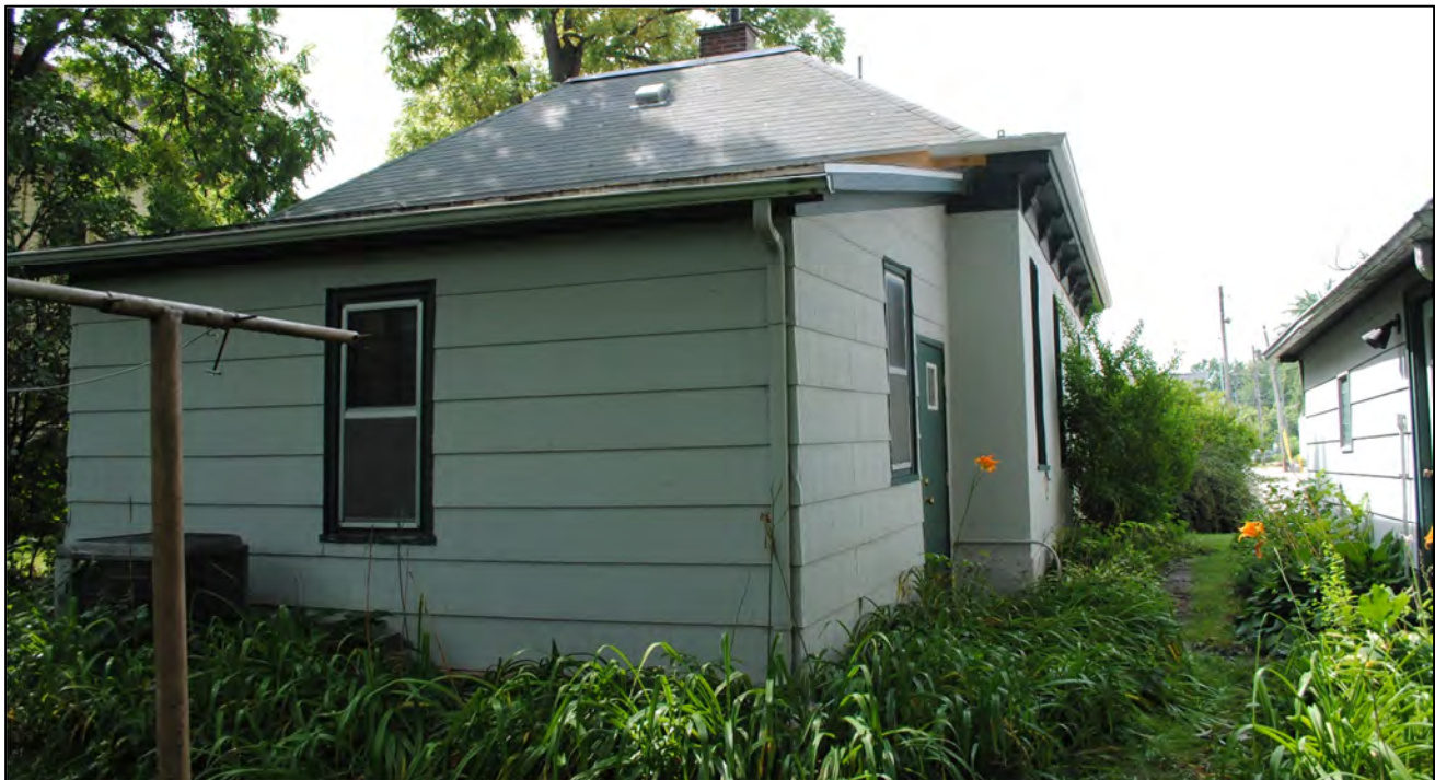
Figure 22. Rear and West side of 509 W. 1st Street looking SSE. Photograph taken 08-07-2018 by Tallgrass.
