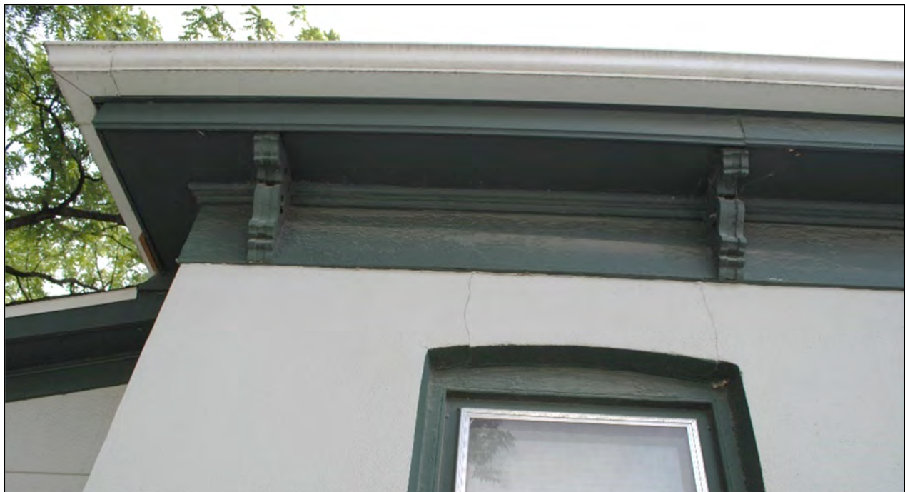
Figure 19. Detail of brackets under the eaves of 509 W. 1 st Street facing West. Photograph taken 08-07-2018 by Tallgrass.
