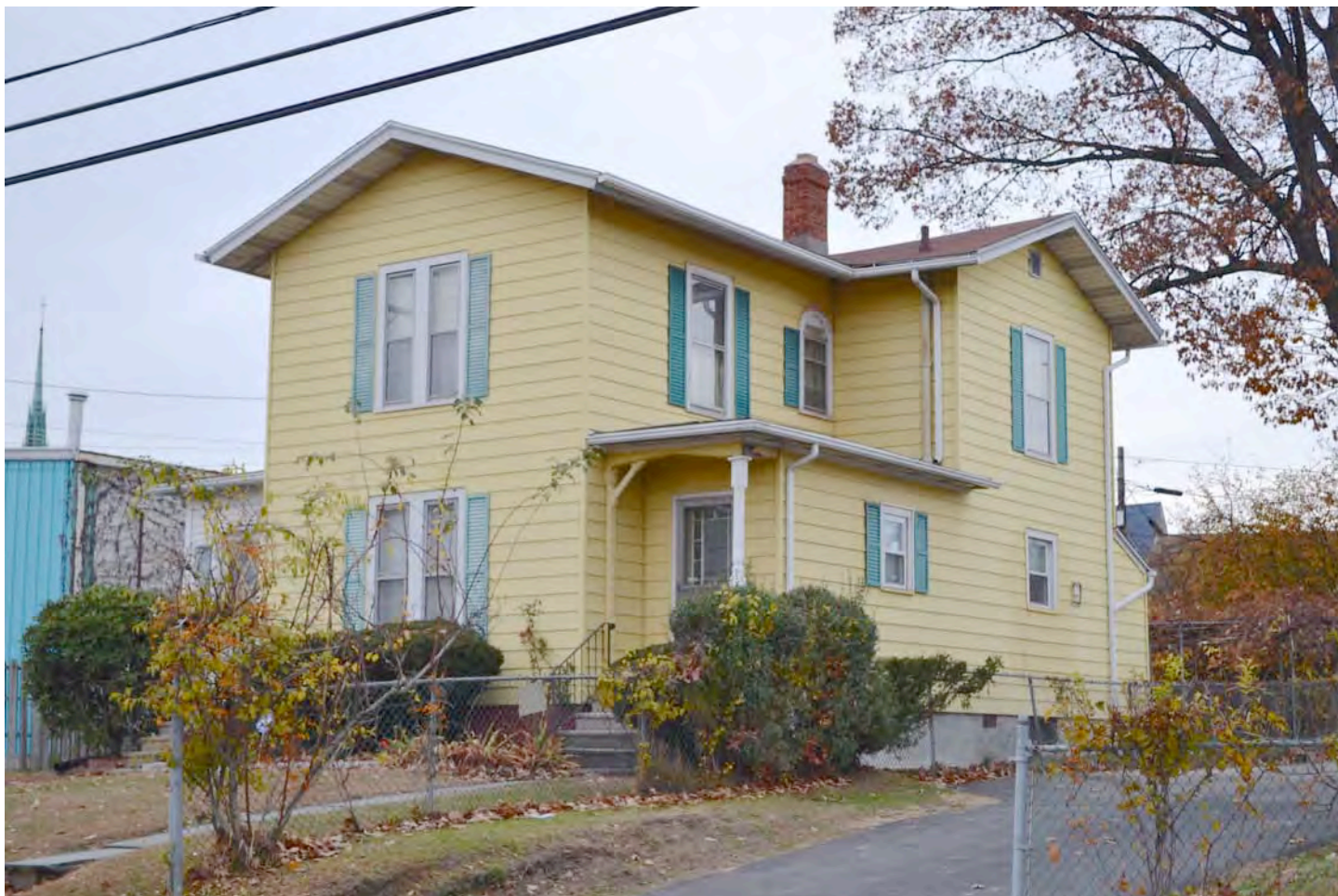
East (front) and north (side) elevations of 61 Francis Avenue (c. 1875). Camera facing southwest. Photograph 39 of 58.
