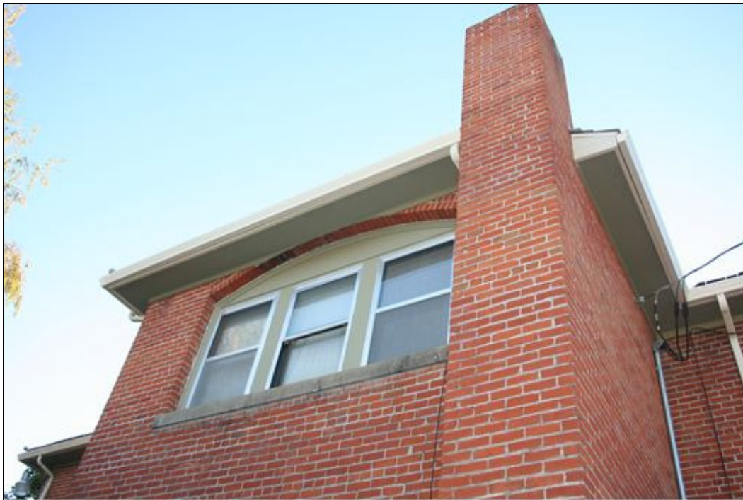
Photo 6 of 14: East façade, looking southwest at large arched rear window in center wing.
