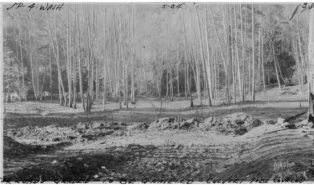
Bowman Bay Parking Area (ID#21) under construction, staked and roughly graded, view to north.
