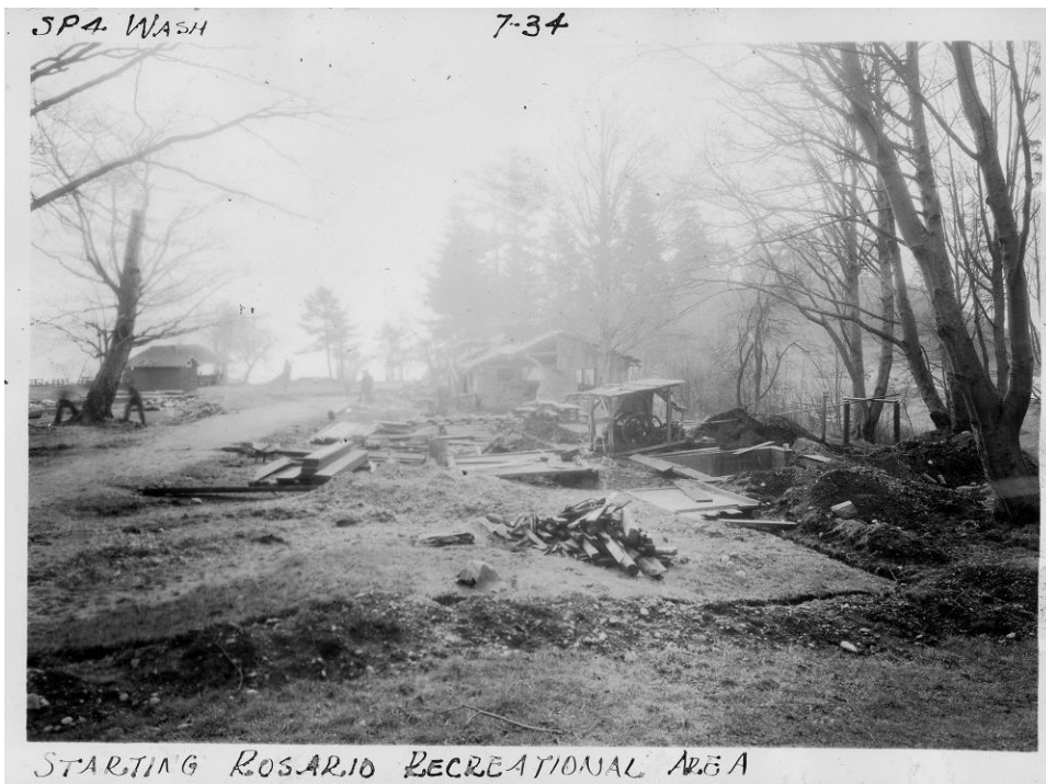
Overview of Rosario area during construction. Community Kitchen (ID#1) in center background, excavation for Pump House (ID#2) in right foreground.
