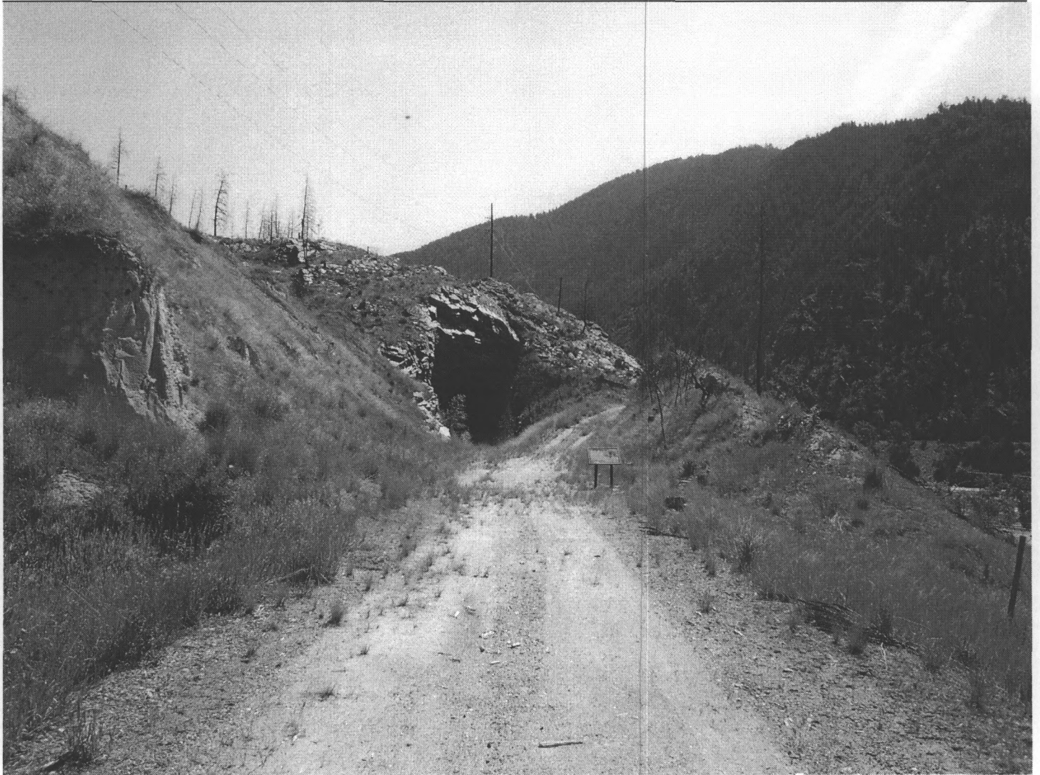
Photo 0028. Section 5. Milwaukee Road Railroad grade. West portal, Tunnel 18. View to east-northeast from western terminus of Section 5.
