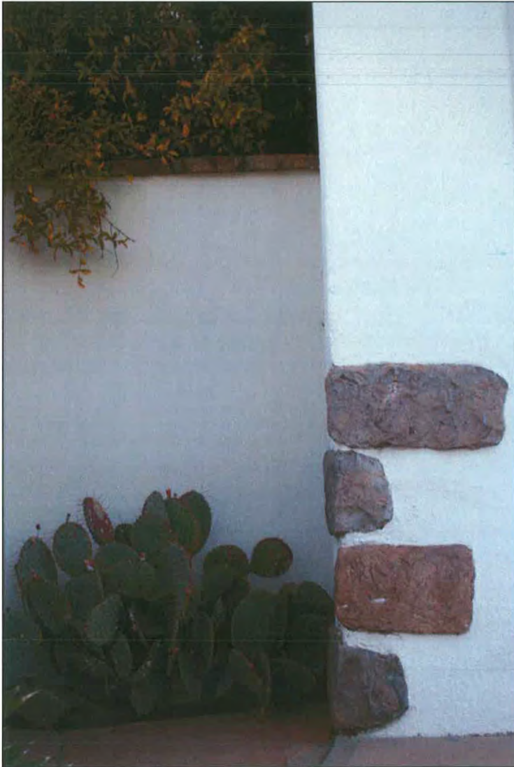
Photograph 7 of 13. Looking west, east elevation, corner stone detail.
