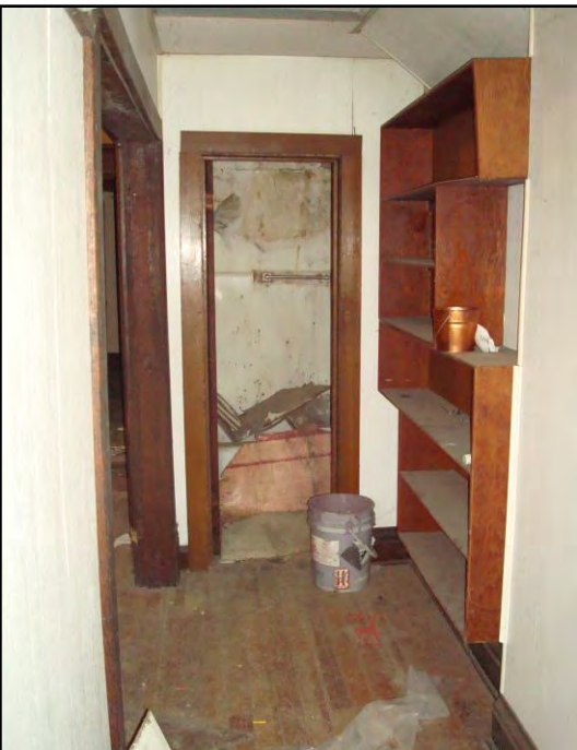
Photo 10. Hallway from entry to bathroom, first floor interior, large built in shelf to west, dining room to east.
