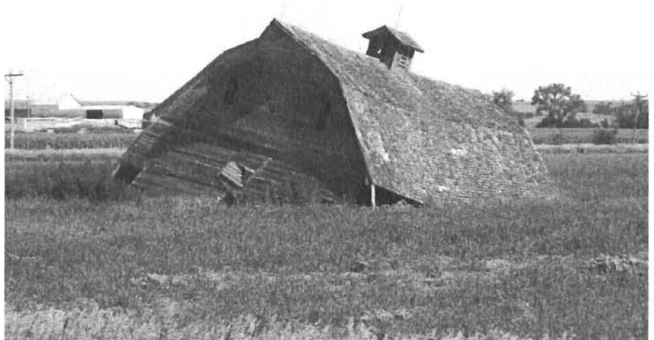
Figure 2: Collapsed Barn in Rooks County. Brenda Spencer.
