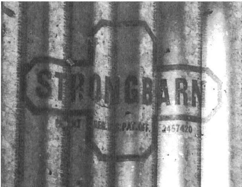
Figure 36: "Strongbarn" was one brand name of corrugated metal used on barns and other agriculture-related structures. Brenda Spencer.
