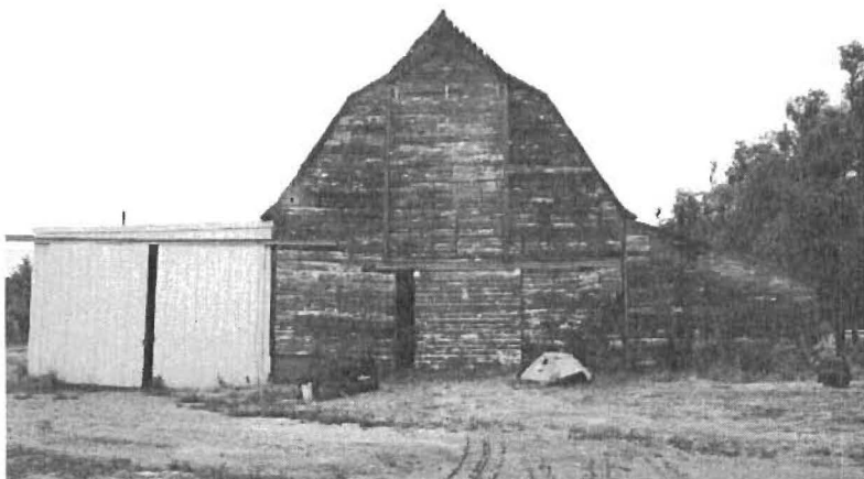
Figure 70: Inappropriate barn addition, Graham County. Brenda Spencer.
