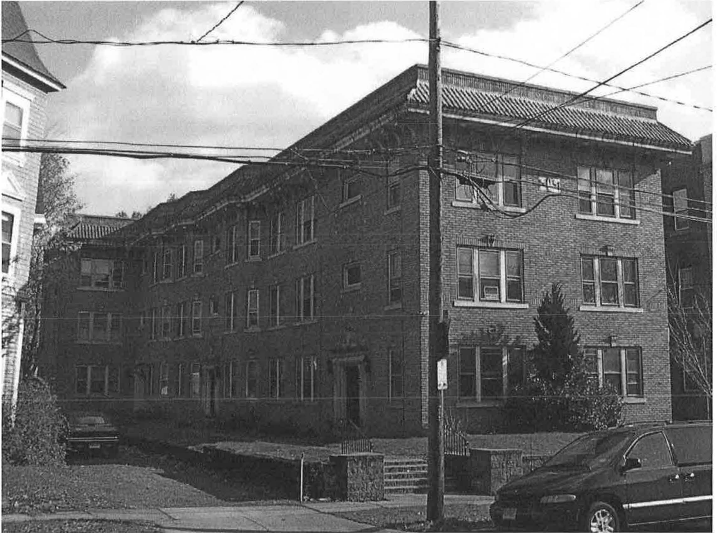
West (front) and north (side) elevations of 28-32 Girard Avenue, 1922, showing façade, roof, entry, and window details.
