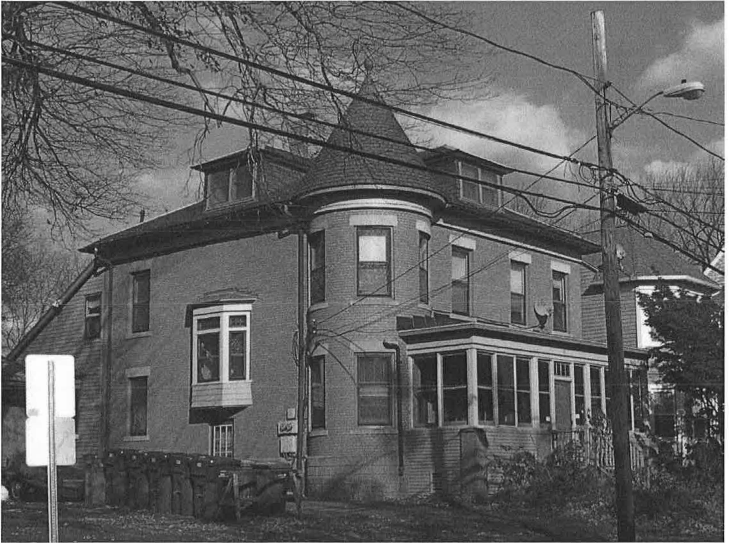
South (front) and west (side) elevations of 18 Warrenton Avenue, 1909, showing façade, roof, porch, and window details.
