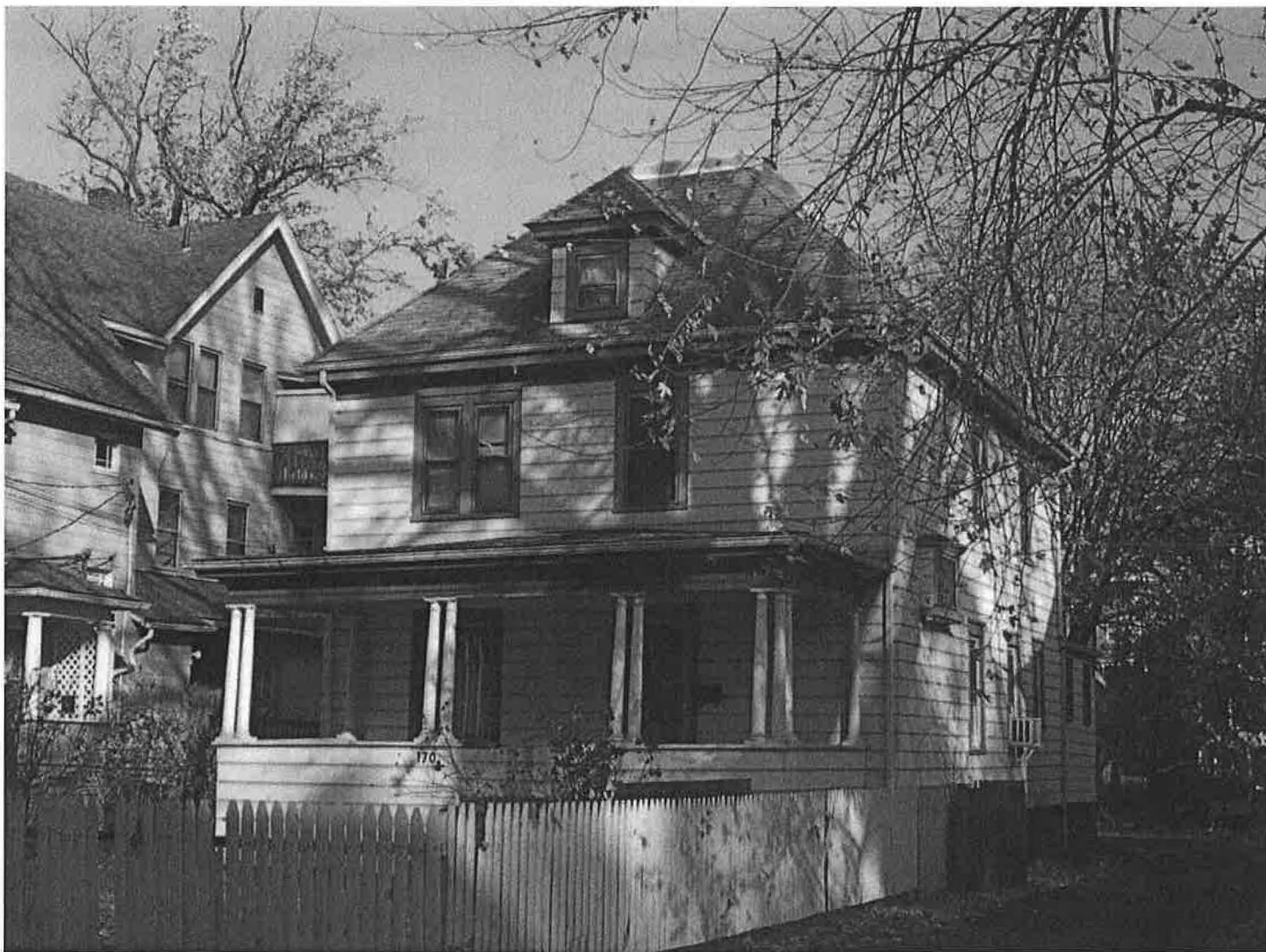
West (front) and south (side) elevations of 170 South Whitney Street, 1901, showing façade, roof, porch, and window details.
