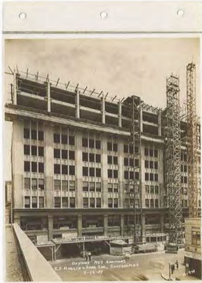
Figure Q. Dayton's Department Store expansion, July, 1937. Photo courtesy of the Minnesota Historical Society.
