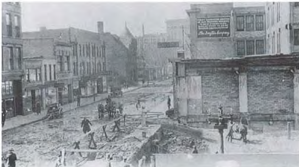
Figure N. Excavation for new addition, c. 1910. Photo courtesy of the Minnesota Historical Society.
