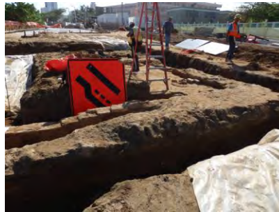
Figure 39. Excavations during the construction of the Paseo de Puerta de Tierra, Puerta de Tierra Historic District, San Juan de Puerto Rico, 2014-2015, Mr José López.
