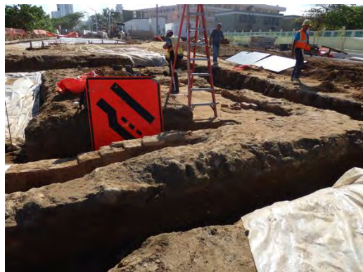
Figure 40. Excavations during the construction of the Paseo de Puerta de Tierra, Puerta de Tierra Historic District, San Juan de Puerto Rico, 2014-2015, Mr José López.
