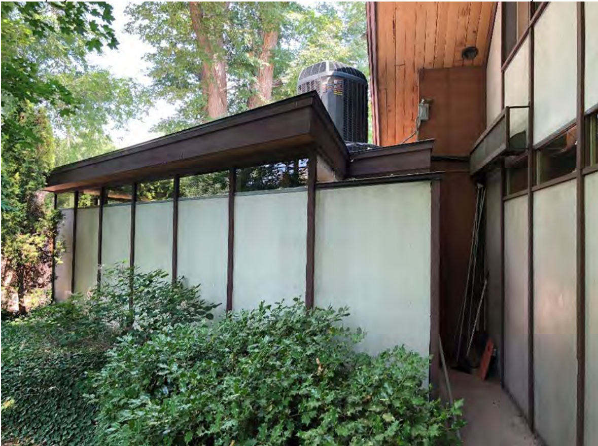
Figure 25 View of shop addition, looking north. Northwest elevation appears to the right in the frame. 39
