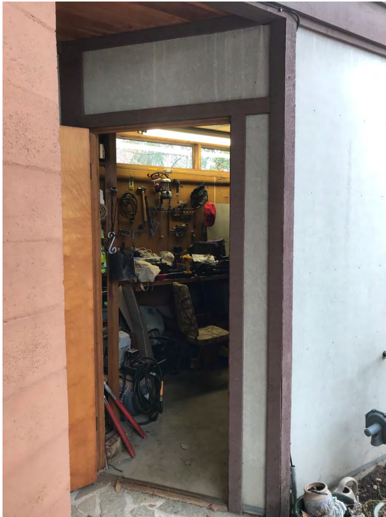
Figure 26 Photo of entrance to shop addition. Photo taken from northwest patio/Zen Garden, looking southwest.
