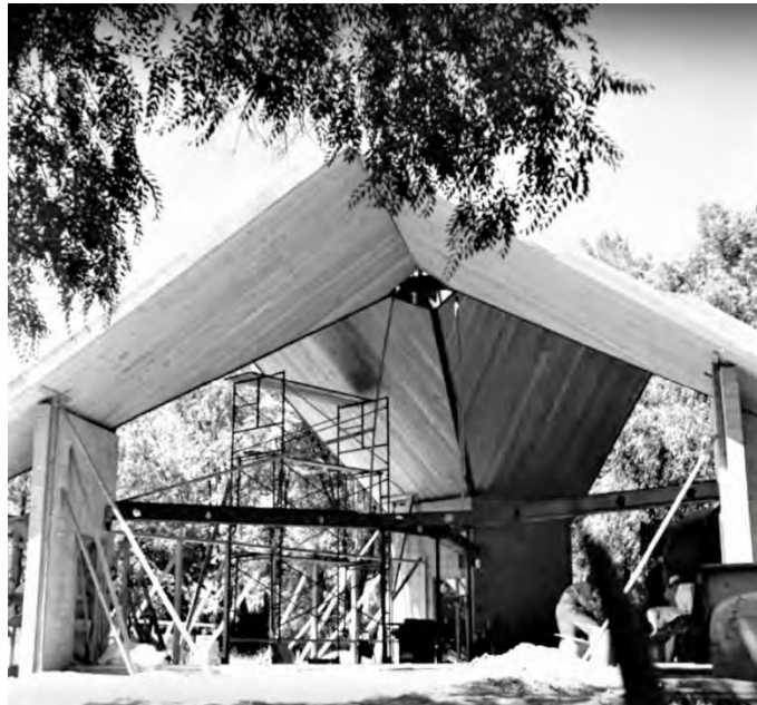
Figure 4 Photograph taken during construction in 1958, showing construction of roof structure containing the truss deck system. 14 Also depicted are corner walls which feature the building's three entrances. These structures remain in place today unaltered from original construction.
