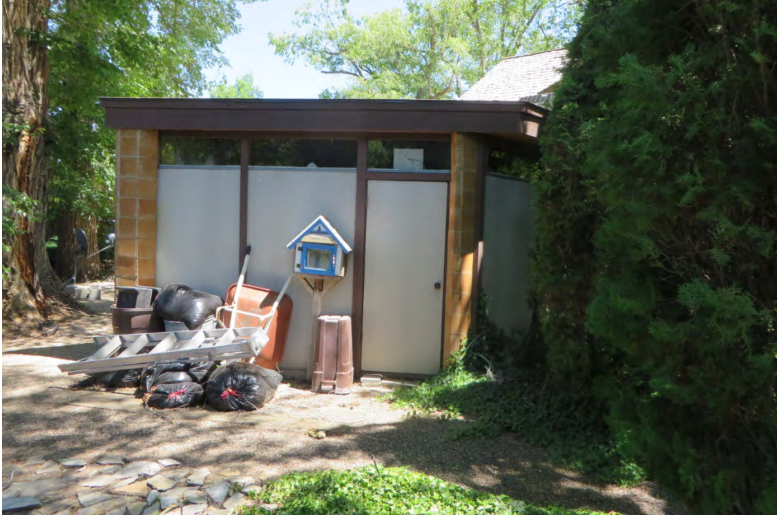
Photo 15 West elevation of Shop Addition, looking east, roof structure of main house in background.
