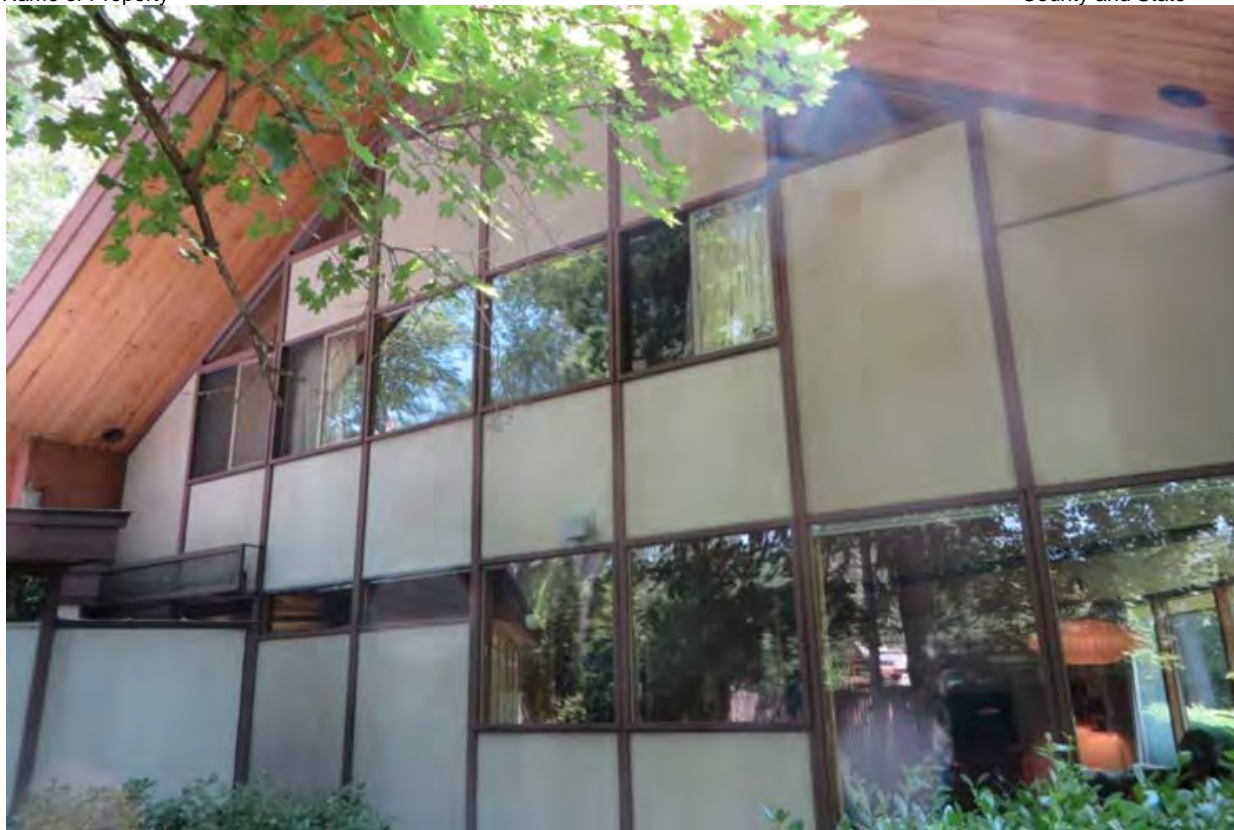
Figure 11 Northwest Elevation; photograph taken looking east. Shop addition located towards lower left of frame, skewing the view of elevation's Cemesto board and window configuration. Window configuration varies slightly from original plan, however, general window configuration and all Cemesto boards pictured here are original to the house. Interior spaces depicted include first-floor kitchen and dining room, and second floor master bedroom. 25
