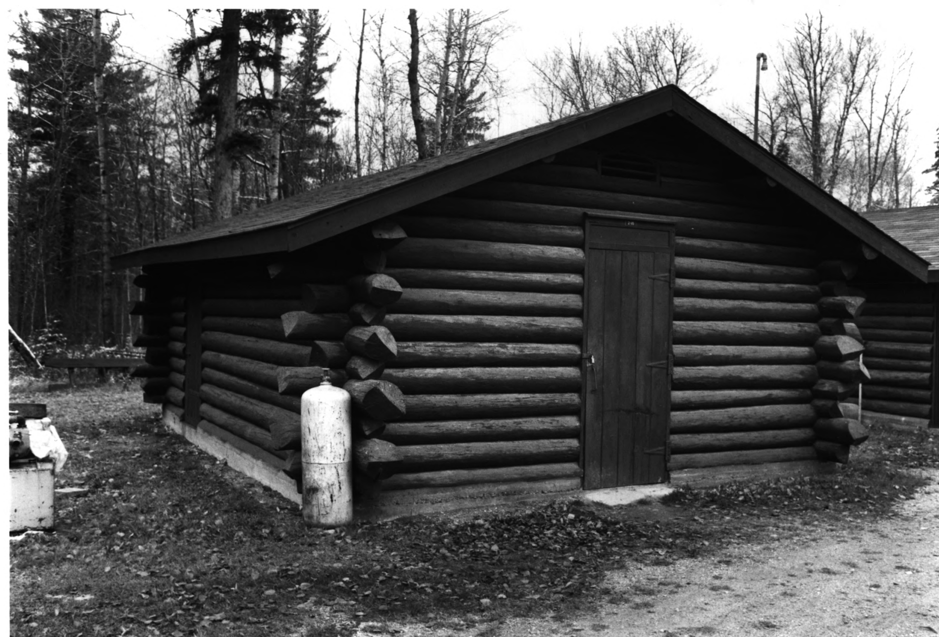
SCENIC STATE PARK - CCC / RUSTIC STYLE SERVICE YARD ITASCA CO., MN BLDG # 4 PHOTO I.D. 09120 # 5
