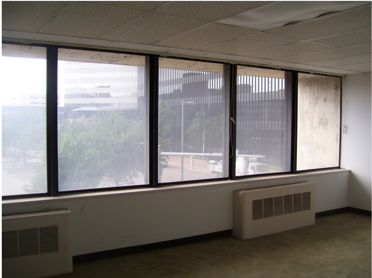
Photo #4 (TX_HarrisCounty_MelroseBuilding_photo_0004) Interior, typical floor on south elevation, replacement windows, view south.
