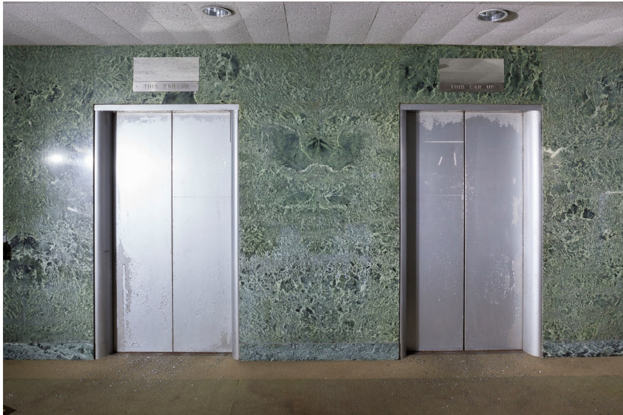
Photo #10 (TX_HarrisCounty_MelroseBuilding_photo_0010) Ground floor elevator lobby; Detail elevators, camera facing west
