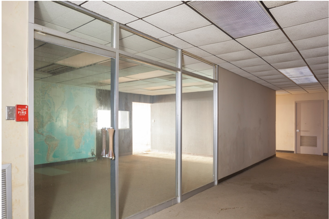
Photo #14 (TX_HarrisCounty_MelroseBuilding_photo_0014) Typical upper floor “blown out” elevator lobby, camera facing southeast
