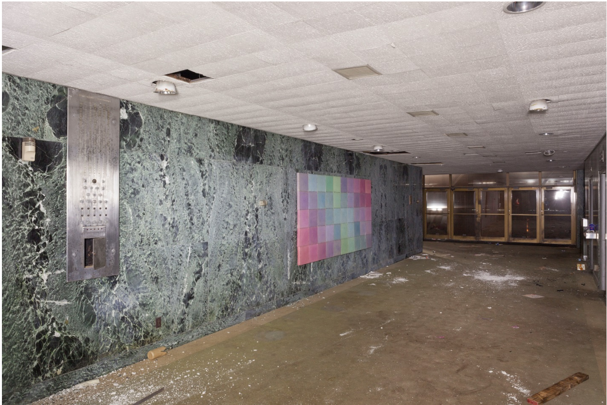
Photo #9 (TX_HarrisCounty_MelroseBuilding_photo_0009) Ground floor elevator lobby; view towards street; E wall on left, camera facing south
