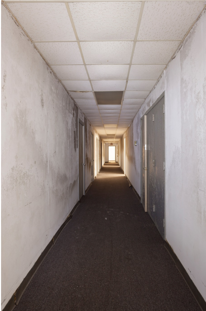
Photo #13 (TX_HarrisCounty_MelroseBuilding_photo_0013) Typical upper floor long corridor from elevator lobby to rear fire stair, camera facing east
