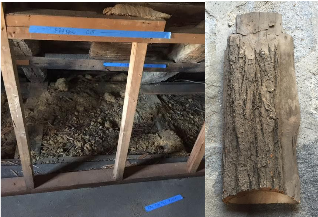
Figure 16. Chestnut lath nailer(s) in situ (left) and removed (right) from western bedroom 2016.
