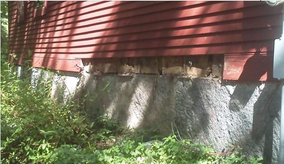
Figure 15. West elevation of main building during restoration. In foreground, visible vertical planking secured to sill atop formal curbstones. View northeast.
