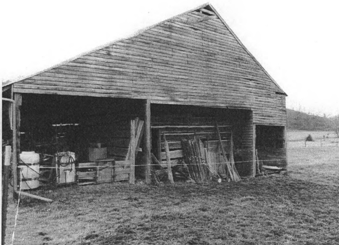
Figure 21. Detail of the northern log crib of the cantilever barn at Maden Hall (D. Brock, 01/2009).
