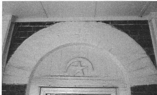
Figure 3. The main entrance is surmounted by an arched opening with a crescent moon and star; an arched fanlight was originally located here before the 1910s fire (D. Brock, upper 03/2009, lower 01/2009).
