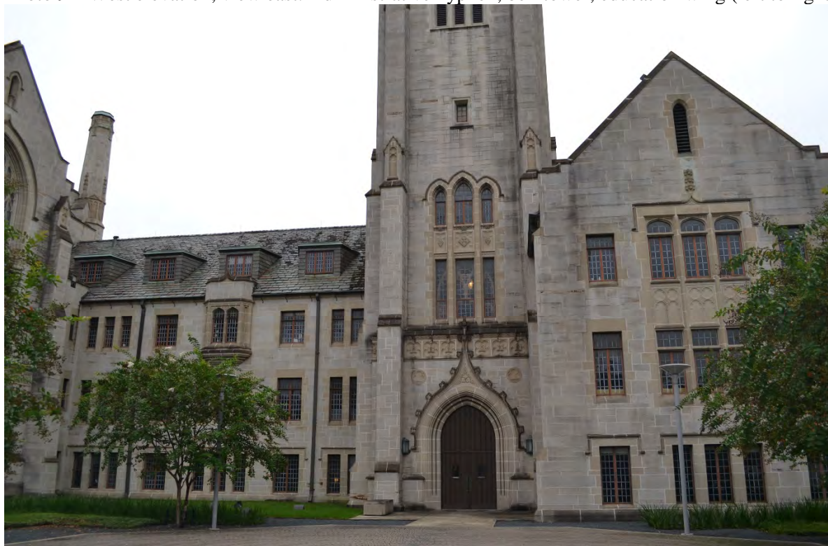
Photo 9 – West elevation, view east. Administrative hyphen, bell tower, education wing (left to right).
