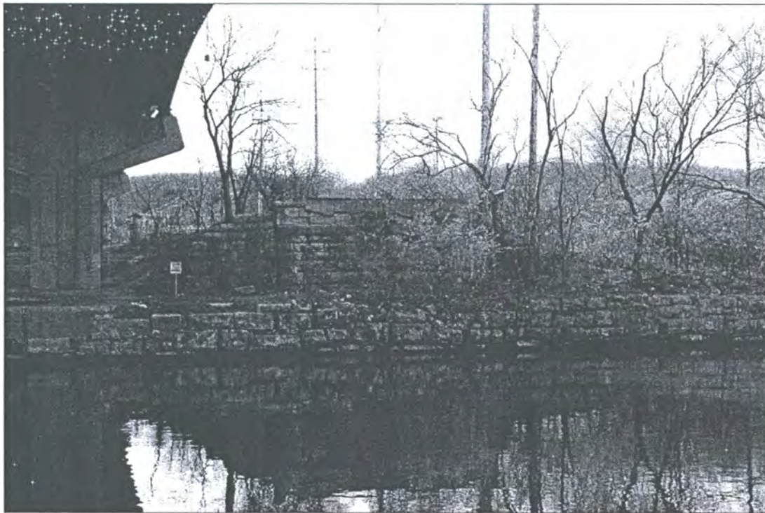
Figure 7: Laid-up limestone walls on the left descending side in the rock segment of the Main Channel south of Willow Springs Road, Cook County, Illinois. View to the southeast. (Photographed by Eyan Bond, April 23, 2009). Digital image on file at Bear Creek Archeology, Cresco, Iowa.
