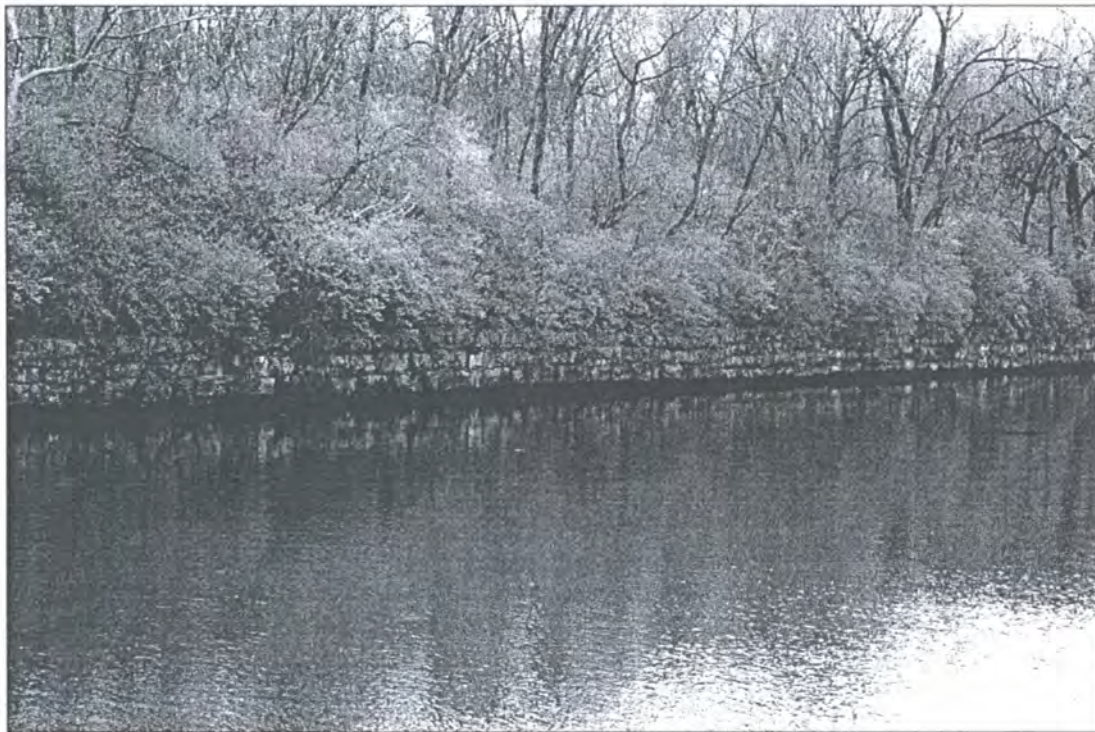
Figure 9: Laid-up limestone walls on the left descending side of the canal in the earth and rock segment of the Main Channel near the Willow Springs Spillway, Cook County, Illinois. View to the southeast. (Photographed by Eyan Bond, April 23, 2009). Digital image on file at Bear Creek Archeology, Cresco, Iowa.
