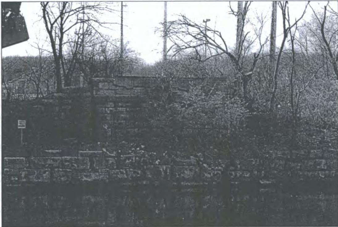
Figure 43: Willow Springs Bridge abutment on the left descending side of the canal, Cook County, Illinois. View to the southeast. (Photographed by Eyan Bond, April 23, 2009). Digital image on file at Bear Creek Archeology, Cresco, Iowa.
