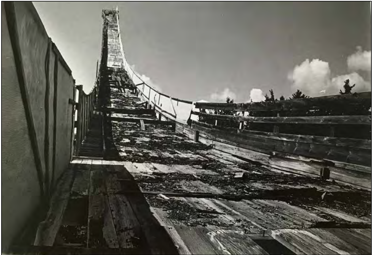
Figure 16. Deteriorated deck of the inrun tower as it appeared in June 1993 (Gagnon 1993).
