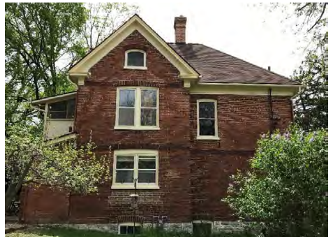
Figure 6 The north side looking south. Note the ground level double window is a reduced replacement. See Figure 7 for a detail view of the juncture of the house and the small addition. May 2018
