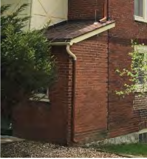
Figure 7 The northeast corner of the house is seen here, with the small east side brick addition to the left. The dark vertical that separates the addition from the house is a tar-like sealant. The foundation appears to be a different stone or masonry type than the body of the house. The bricks have a smoother more finished surface over the earlier red clay bricks of the main house. The latter bricks show press marks. This small addition, c. 1910, houses an interior bathroom and has only a crawlspace underneath. May 2018
