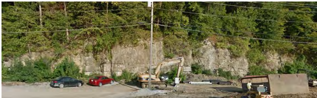
Figure 22 Dubuque Street and the quarry as it appears today. Dubuque Street is undergoing reconstruction in this photo, a project necessitated by severe flooding in 2008. Source: Google on 6/7/2018
