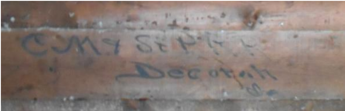
Figure 7 The script on this board is actually upside down as nailed to the wall above the doorway from the freight room to the waiting room, suggesting it was salvaged from elsewhere in the building.
