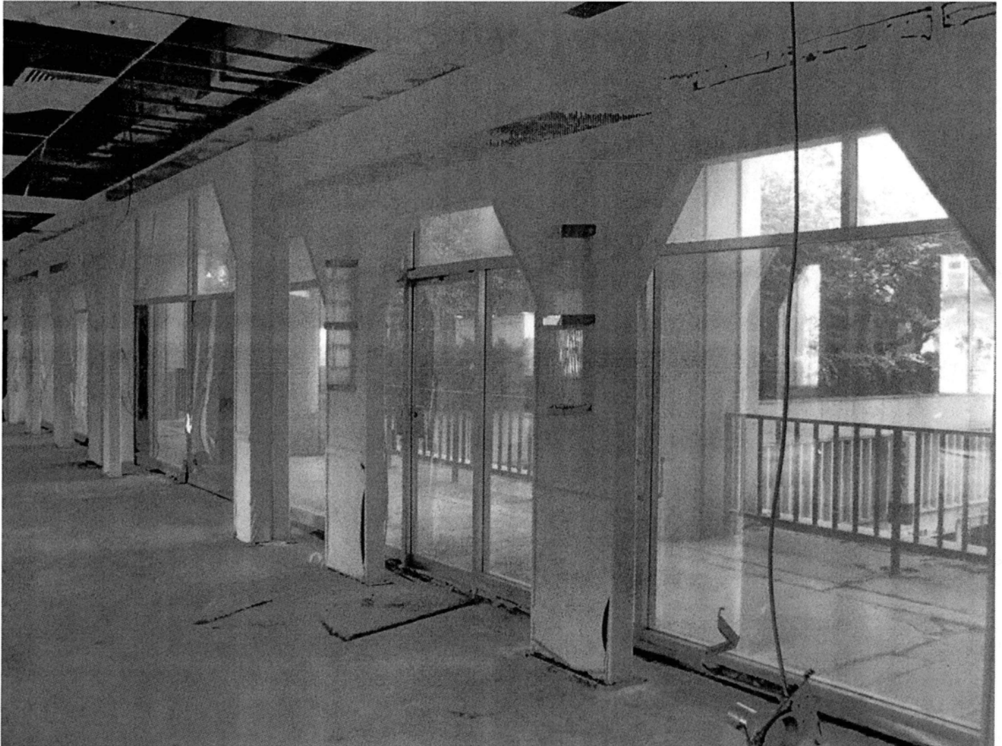
Interior of the third-floor hall, showing floor, wall, window, and ceiling details. Camera facing southwest. Photograph 24 of 28.
