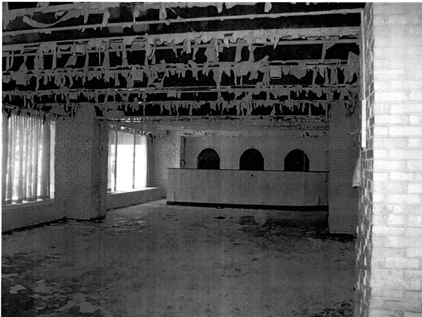
Interior of former "Rib Room" restaurant, showing floor, wall, window and ceiling details. Camera facing southeast. Photograph 20 of 28.
