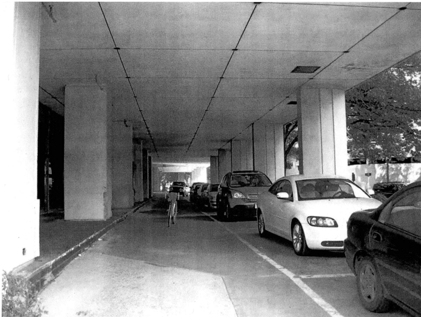
East (front) elevation of hotel from Columbus Boulevard, showing column details. Camera facing north. Photograph 6 of 28.
