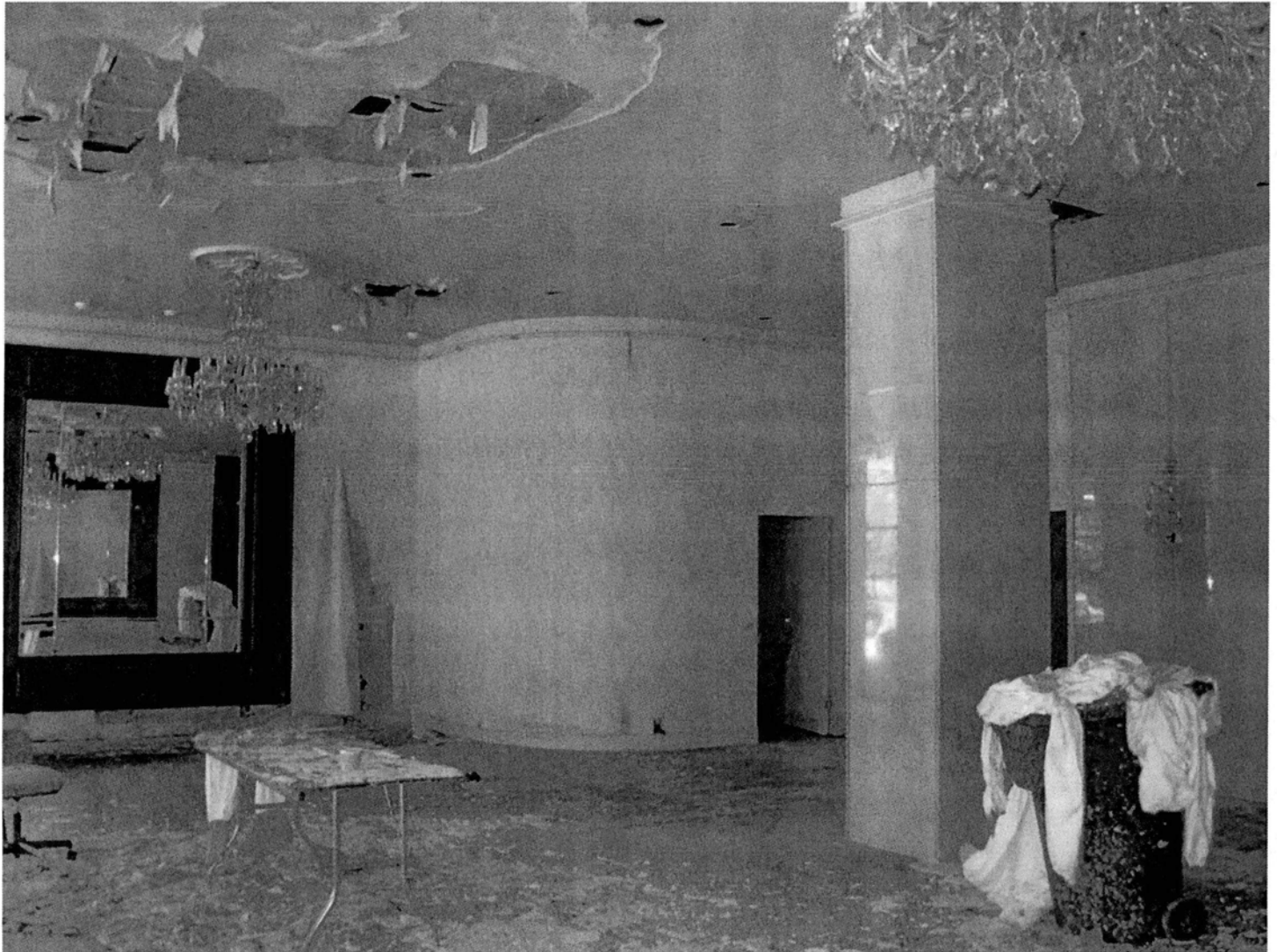
Interior of main lobby, showing floor, wall, and ceiling details. Camera facing southwest. Photograph 16 of 28.
