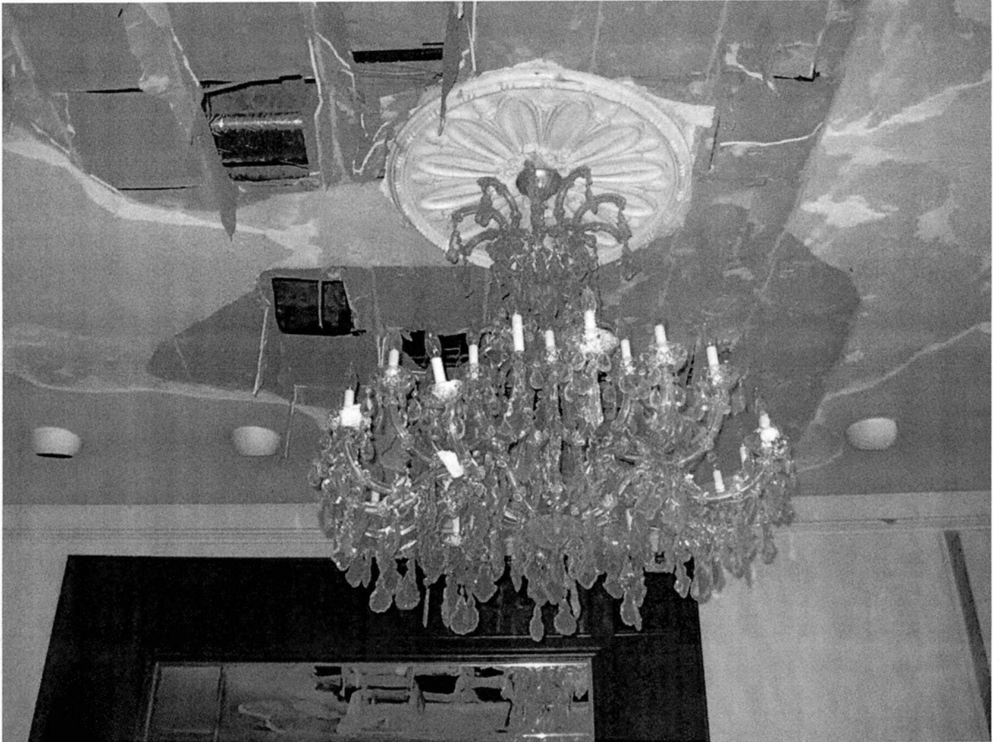
Interior of main lobby, showing ceiling, chandelier, and medallion details. Camera facing south. Photograph 17 of 28.
