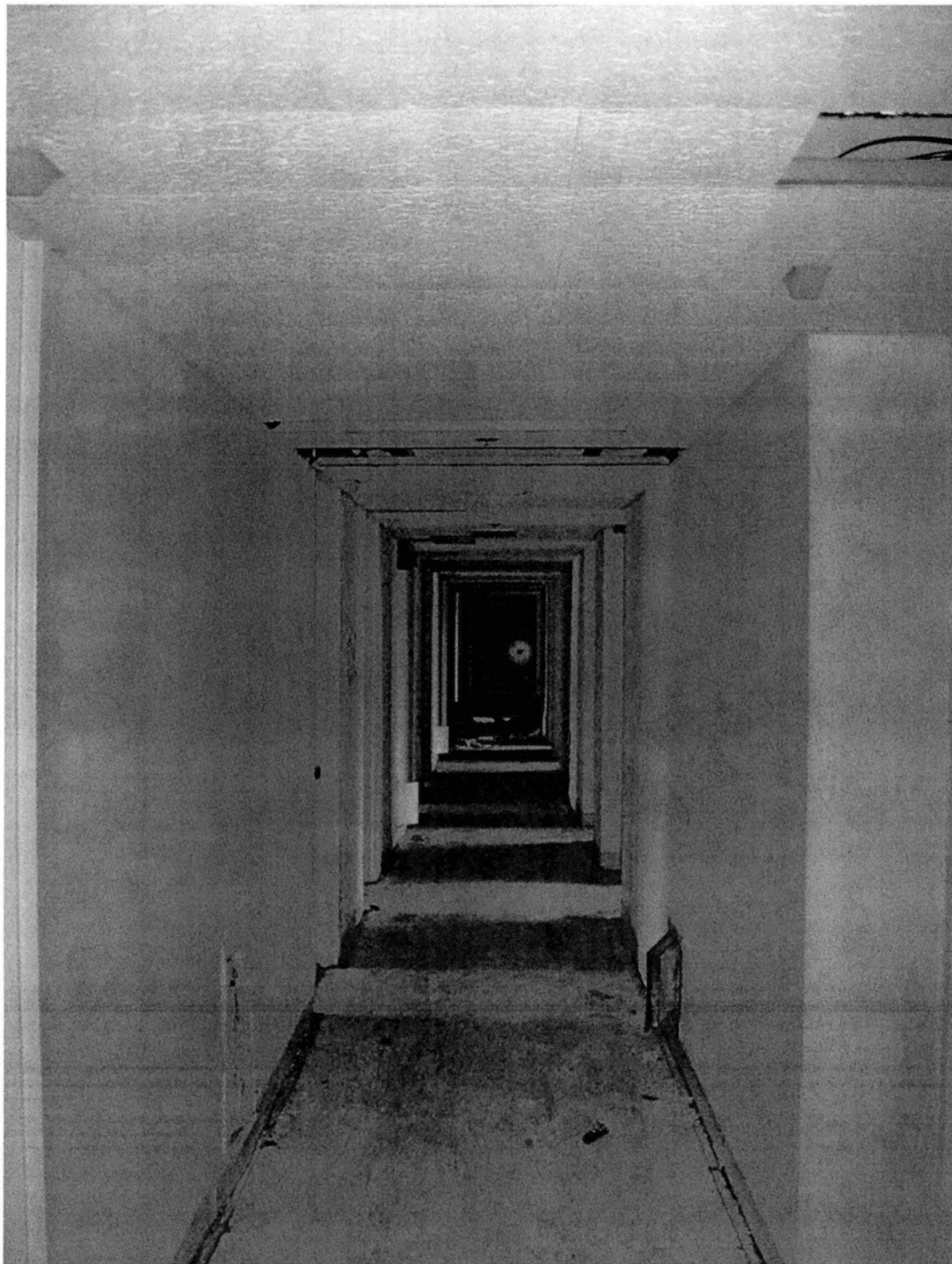
Interior of the fourth-floor corridor, showing floor, wall, and ceiling details. Camera facing north. Photograph 26 of 28.
