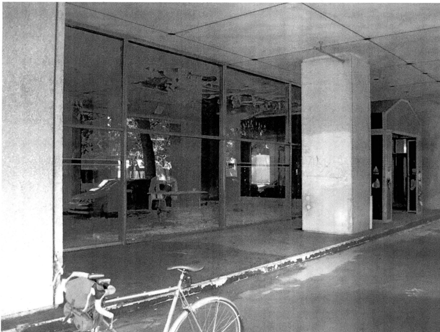
East (front) elevation of hotel from Columbus Boulevard, showing window and wall details of southern block.
