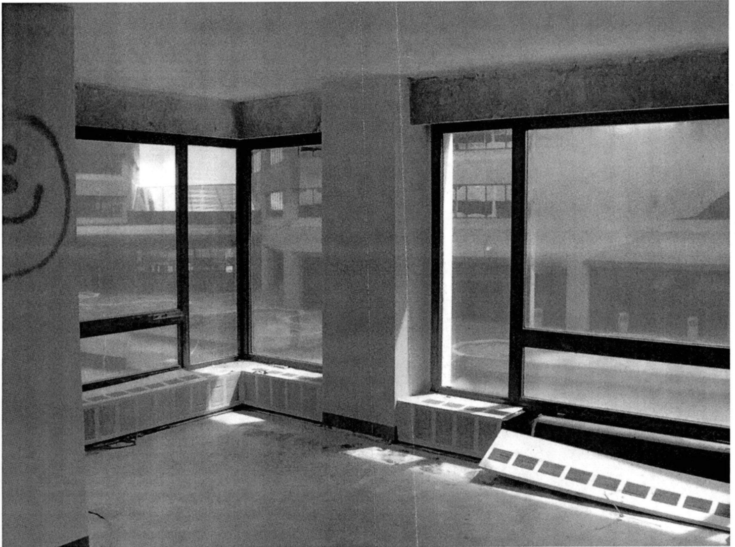
Interior of typical corner guestroom, showing floor, window, wall, and ceiling details. Camera facing northeast. Photograph 27 of 28.
