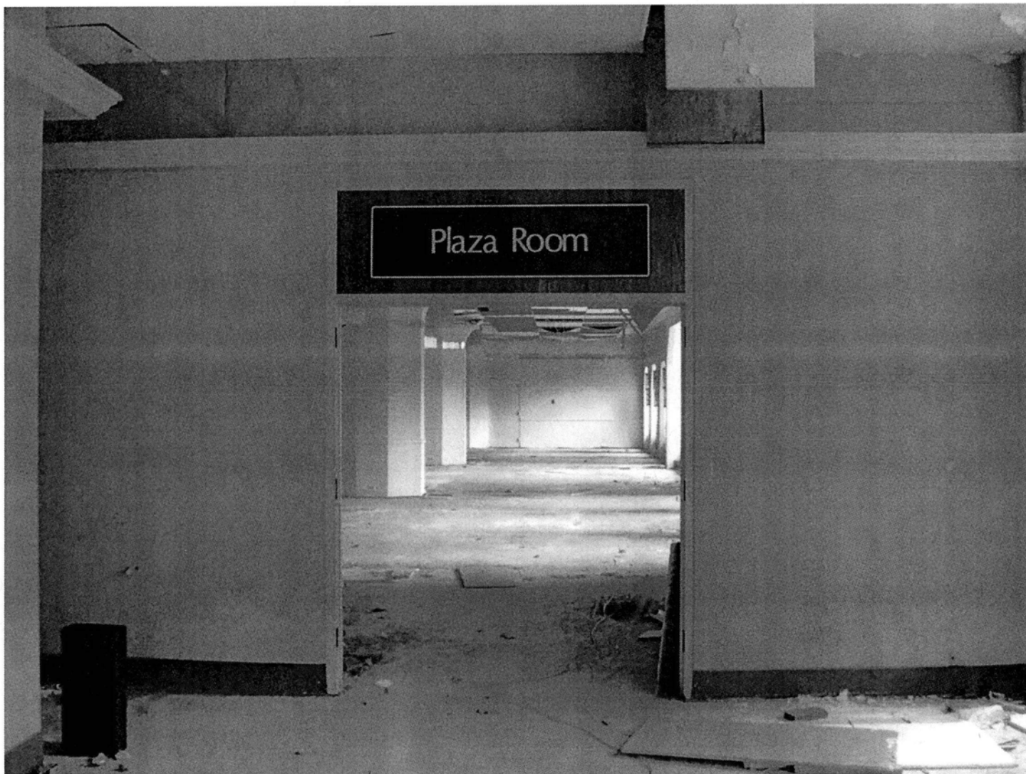
Interior of the third-floor hall, showing floor, column, and wall details. Camera facing north. Photograph 23 of 28.
