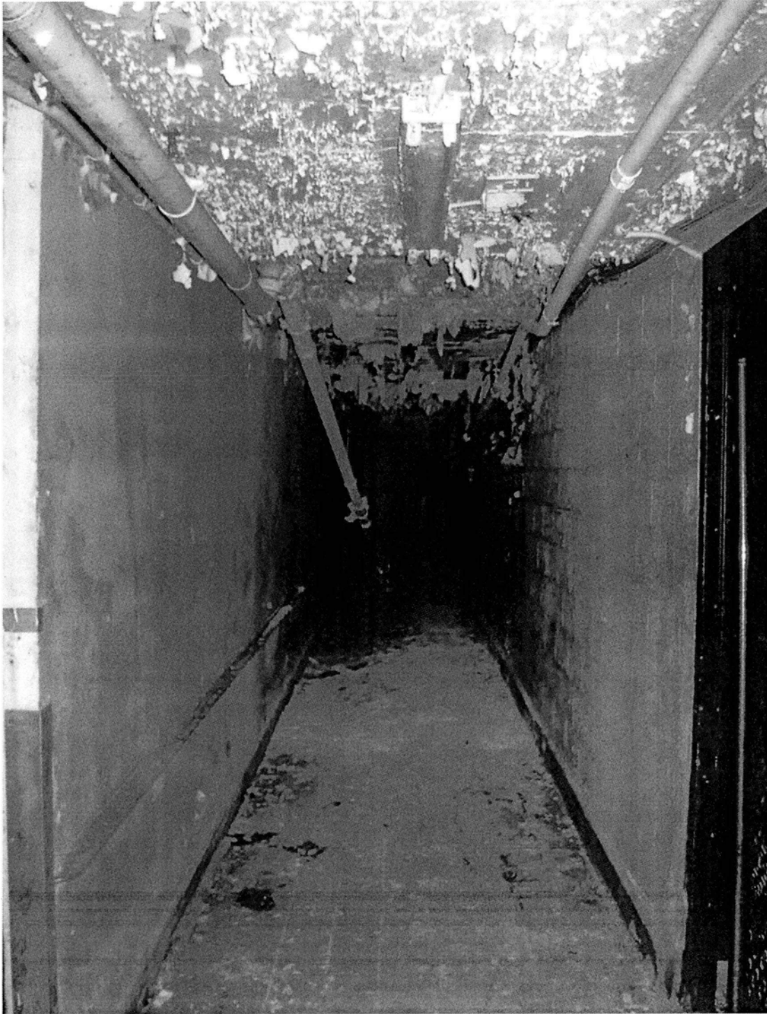
Interior of central food service corridor, showing floor, wall, and ceiling details. Camera facing south. Photograph 21 of 28.
