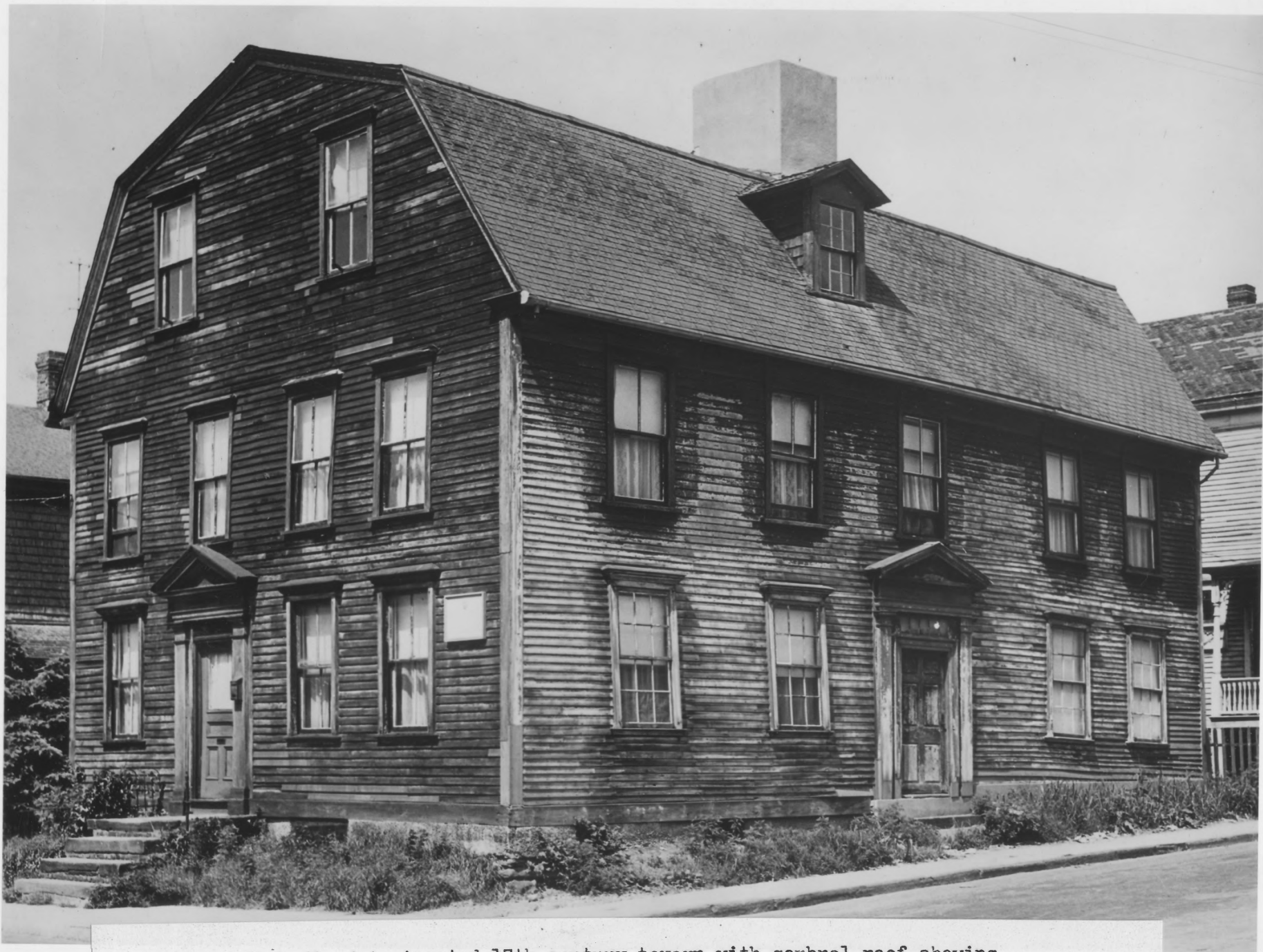
A badly deteriorated 17th-century tavern with gambrel roof, showing modified chimney and windows
