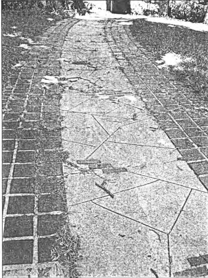
JC 5. 415 N. Jefferson St., 1928. This driveway features easily identifiable work by Julian Cramer and his brothers: incised concrete to resemble tiles and diamond brick insets framed by square brick pavers.
