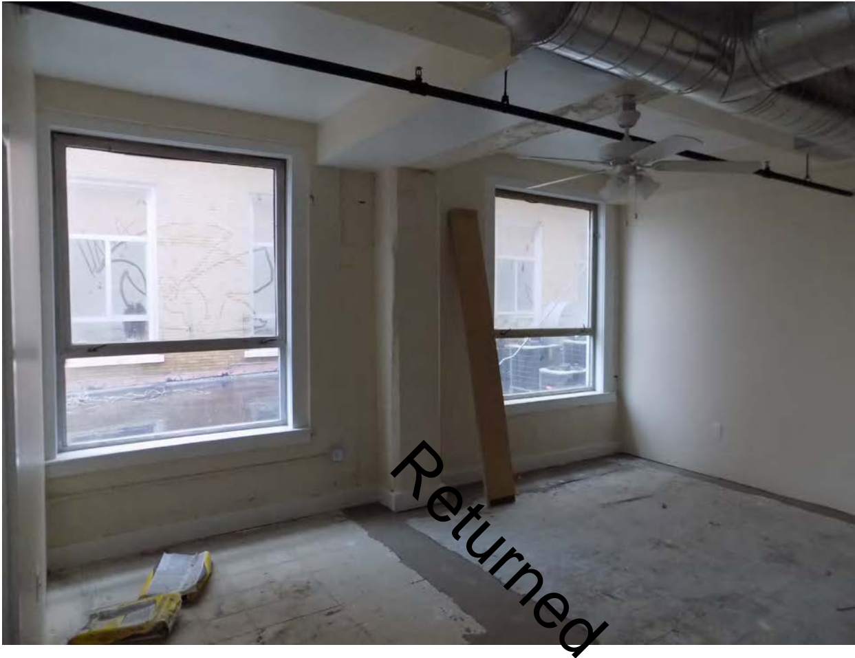
Figure 14: Interior of building showing exposed concrete structural system. Source: Michael Allen photograph taken June 20, 2016.
