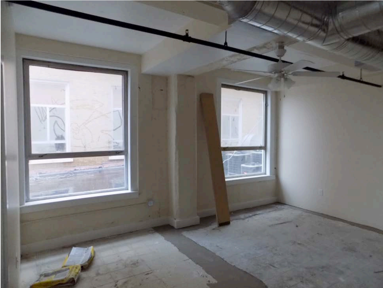
Figure 14: Interior of building showing exposed concrete structural system. Source: Michael Allen photograph taken June 20, 2016.
