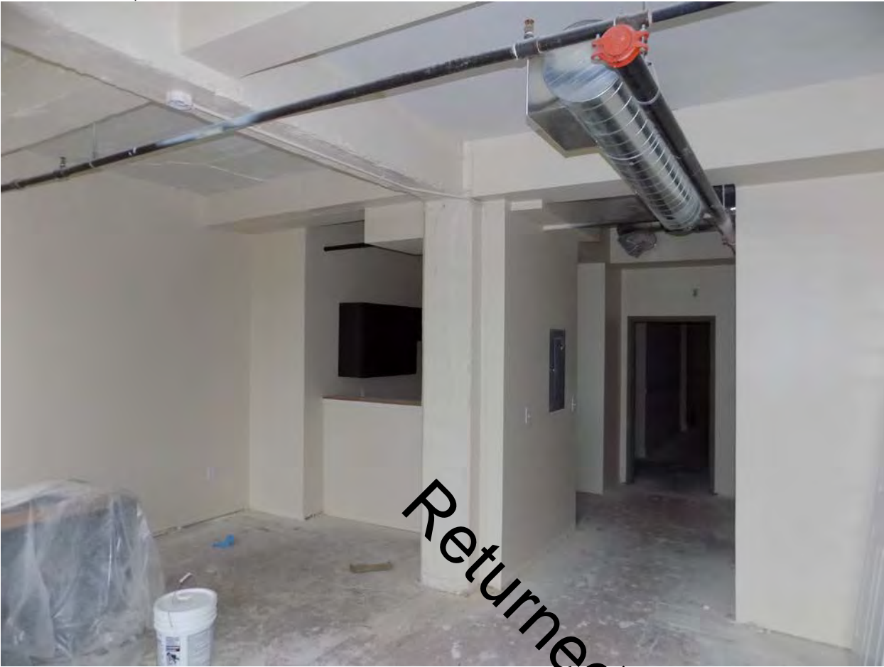
Figure 13: Interior of building showing exposed concrete structural system. Source: Michael Allen photograph taken June 20, 2016.
