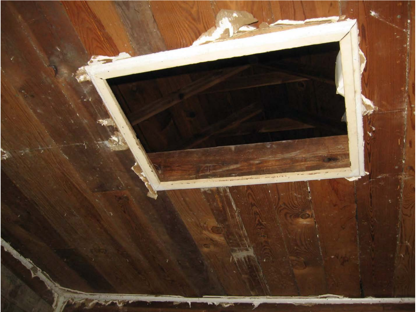
Figure 23. 2009 photo showing the attic opening in the back hall. Image courtesy of Kerry Lincoln.
