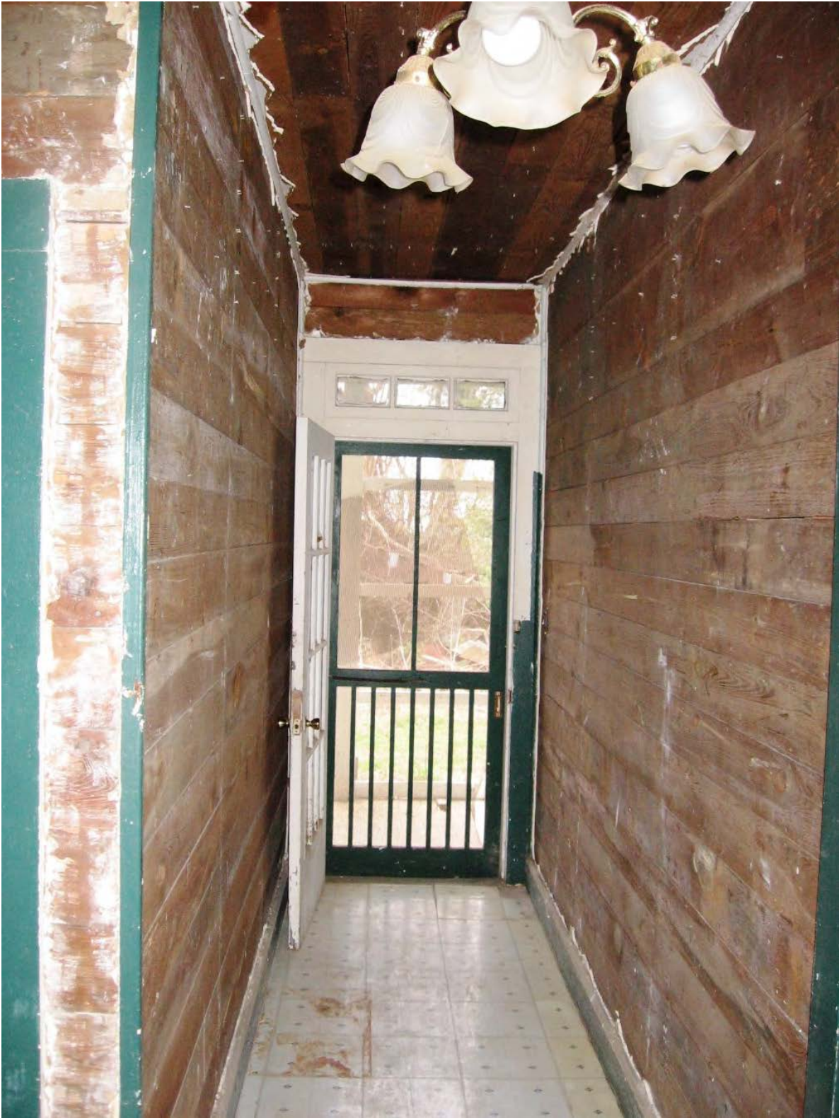
Figure 19. 2009 photo showing the back hall to the outside porch. The kitchen is to the right and bedroom 3 is to the left. Image courtesy of Kerry Lincoln.
