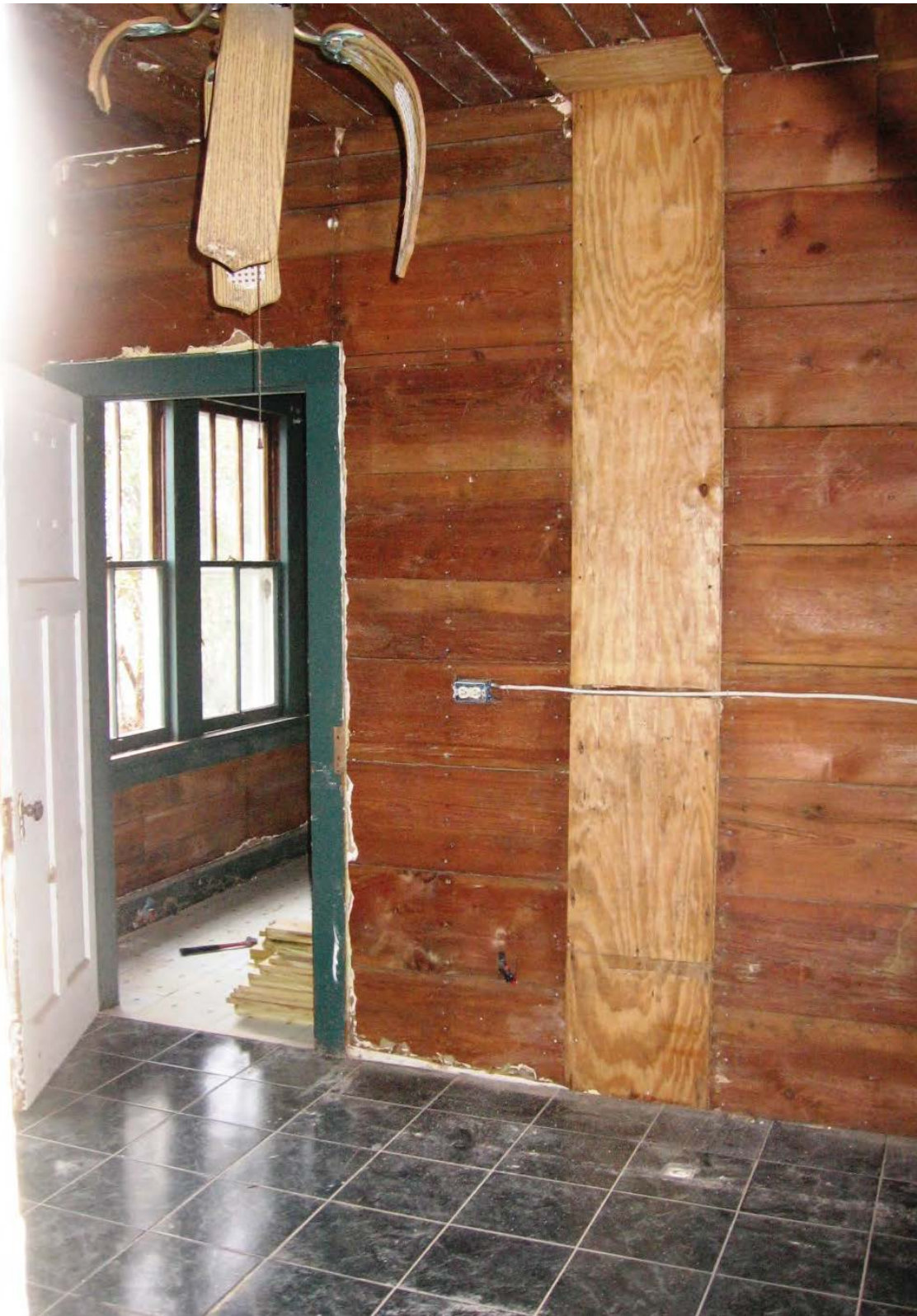
Figure 17. 2009 photograph in the kitchen facing east where the second fireplace was located. The light colored wood was used to fix the walls in the 1940's when this fireplace was removed and a modern stove was installed in the space. Image courtesy of Kerry Lincoln.
