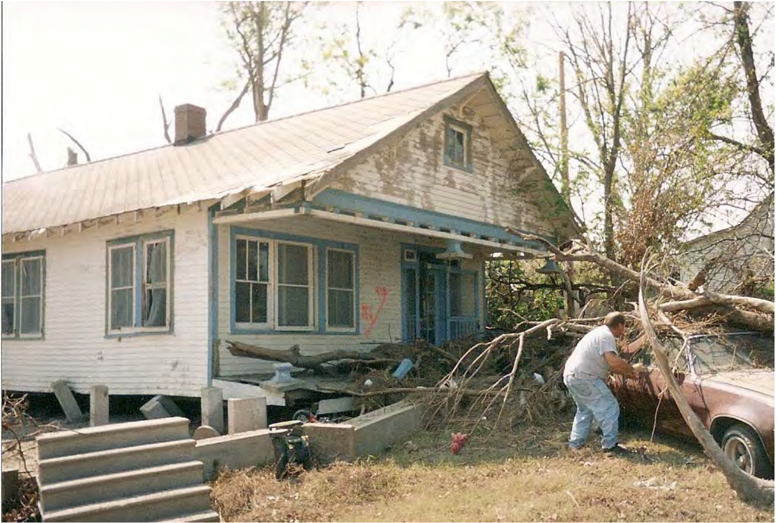
Figure 11. More than a year after Hurricane Katrina the George Lincoln house was still off its piers waiting for workers to help set it back. Two of its three columns on the front were intact. Surprisingly the porch overhang maintained its integrity. Image courtesy of Rod Lincoln.
