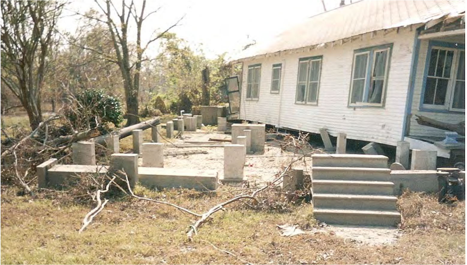
Figure 12. 2006 photo from the front (east) of the house showing the original piers and how much the house floated from its original location. Image courtesy of Rod Lincoln.
