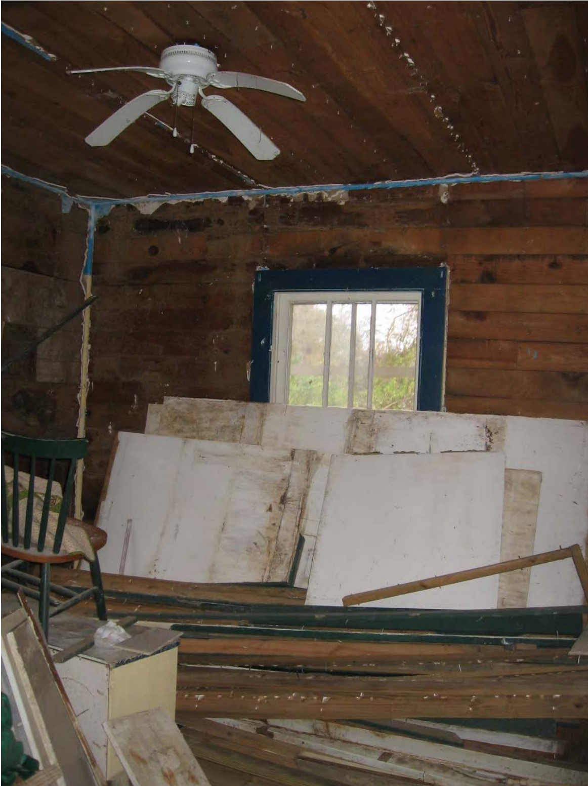
Figure 18. 2009 photo showing the back bedroom. This room was used for staging much of the cypress and hardware during renovation. To the left are two doors. The closest to the window was a closet. The more distant from the window was the entry door from the back hall. The west facing wall has a window looking onto the back porch. The wall behind the photographer is just a long blank wall running parallel with the hall. Image courtesy of Kerry Lincoln.
