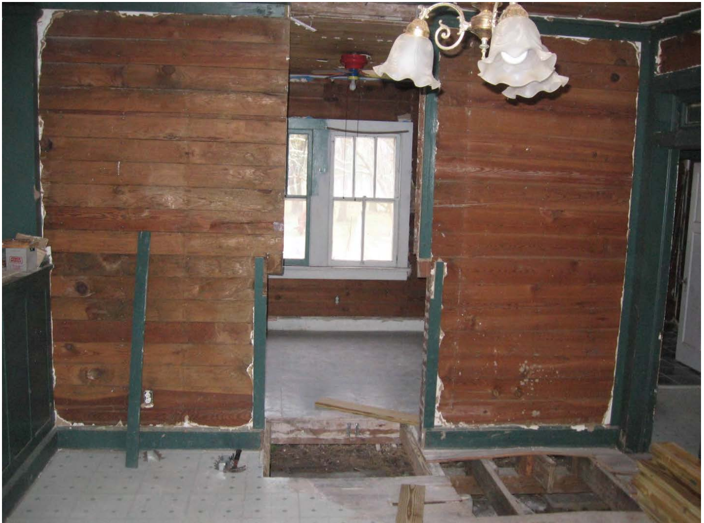
Figure 15. 2009 photograph of the Lincoln House. To the left is the back of a built in book shelf and to the right is the door into the hall from the Living Room. This hole was previously where a fireplace was located between the Living Room and the middle bedroom. The chimney was damaged when the house floated during hurricane Katrina and had to be removed. Image courtesy of Kerry Lincoln.
