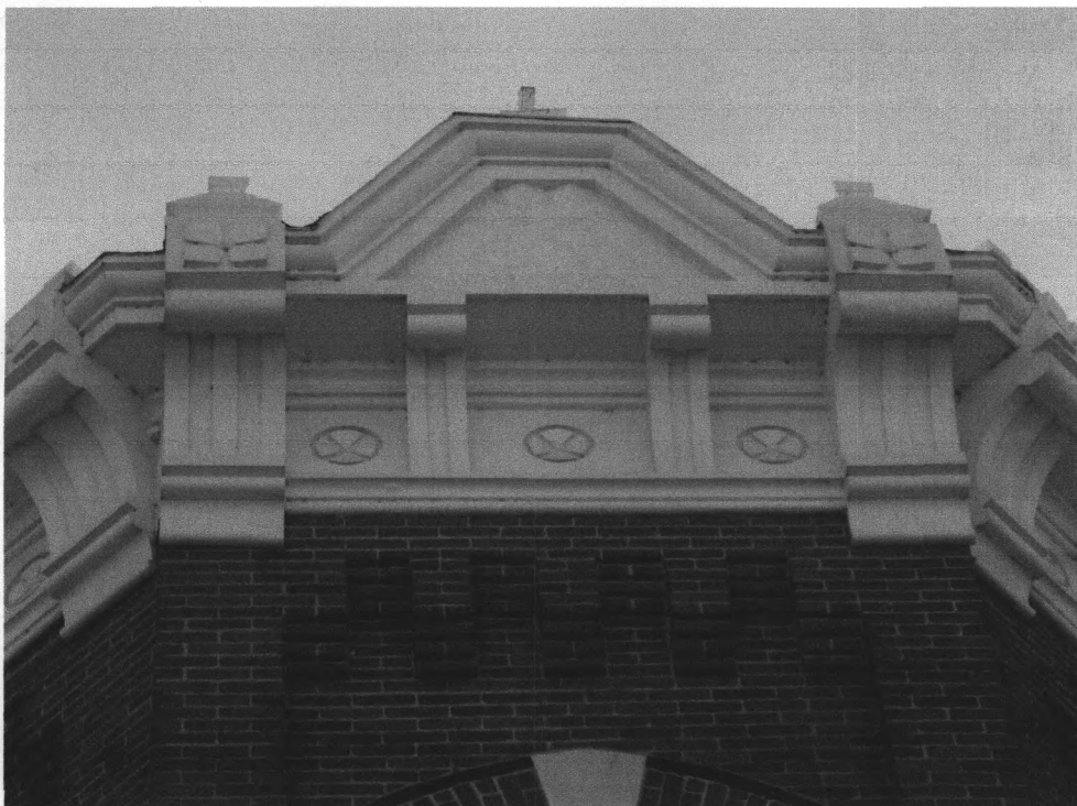
Figure 2 Detail of metal cornice atop the canted corner. Photo by Tallgrass Historians L.C., 2008
