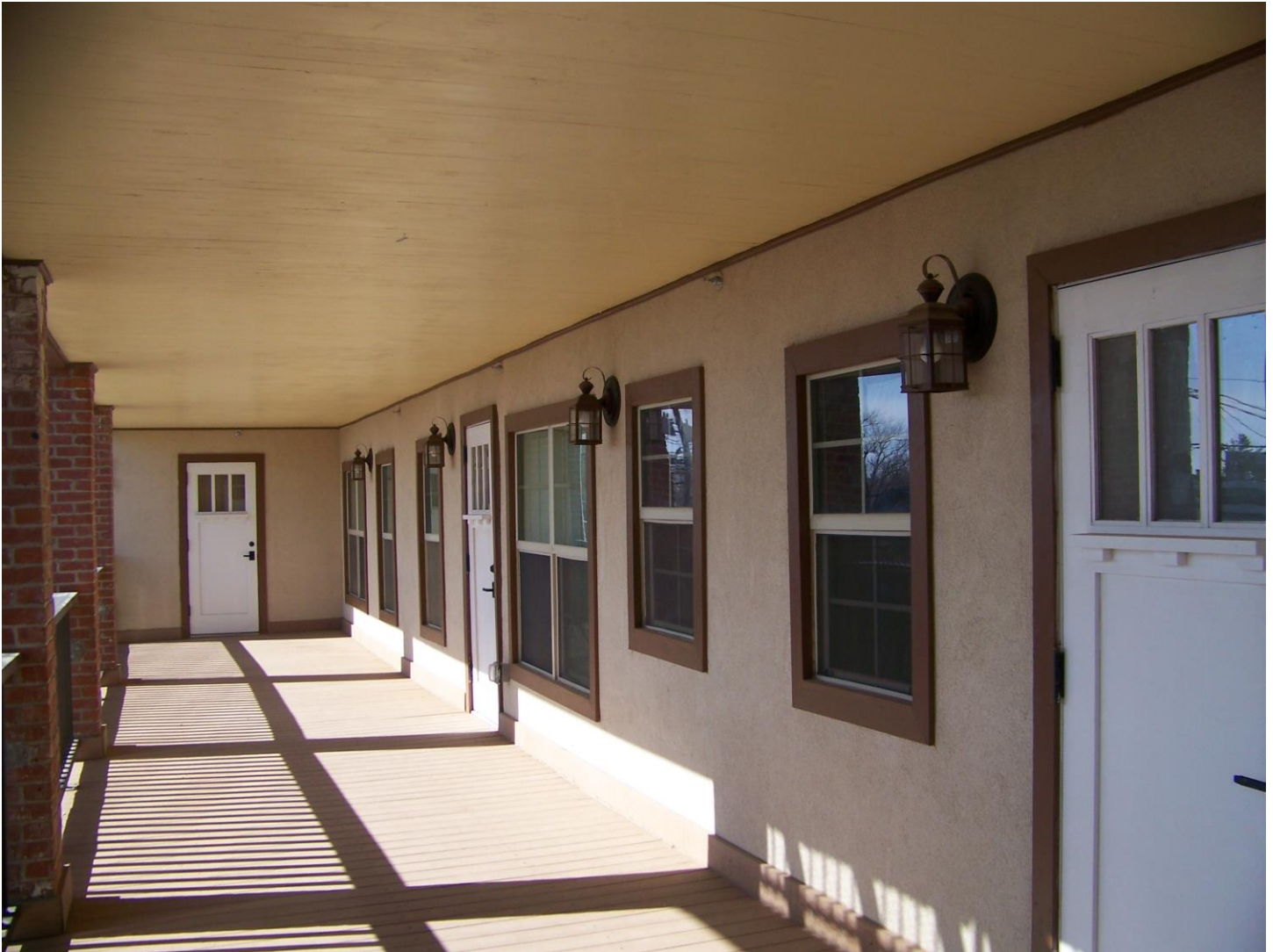
TX_Potter County_Vineyard Manor_0005.tif Rear balcony, second floor, detail. Camera facing approximately south.
