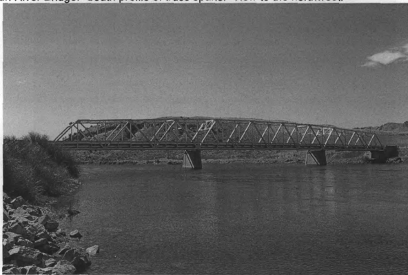
Photo 0004. Missouri River Bridge. North profile of truss spans. View to the south..
