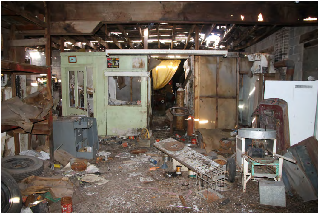
9 of 18. Interior, office (left) and passage to rear radiator service addition (center), photographer facing northeast.
