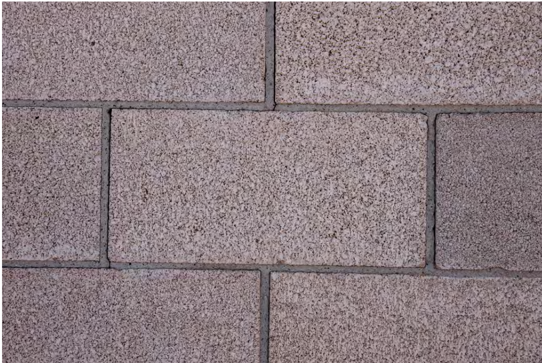
7 of 18. Detail of pumice blocks, north side of radiator addition, photographer facing southeast.
