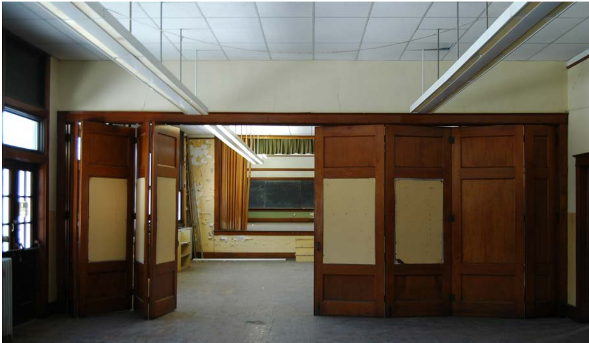
Photo #6 Classroom 1, northeast wall
