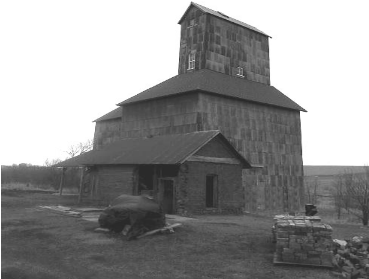
1 of 5. View of the office and the elevator as seen from the northeast. The office is still under rehabilitation. The elevator and annex are nearly complete. (Ross Iowa Grain Elevator, Ross, IA. Audubon County, Iowa. Photographer, Robert Nelson, owner. Photo taken March 2017.)
