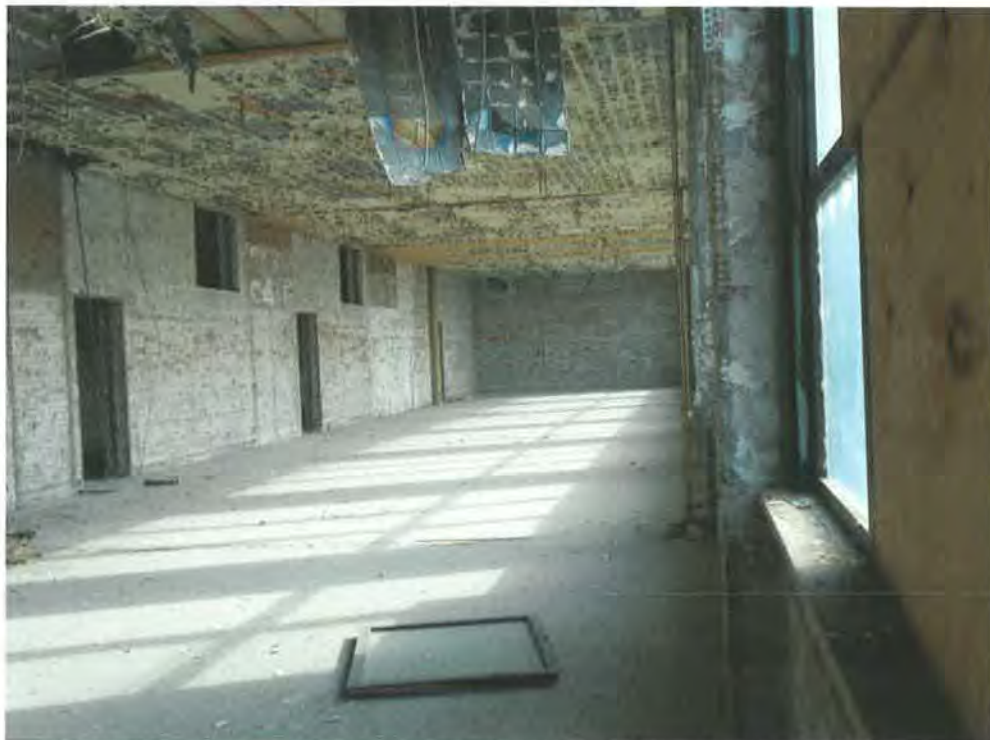
Second floor class room with both original and later room partitions gone. Note the high, newly exposed corridor window openings at left and the decorative metal ceiling that spans the length of this space. The windows on the right are at the front of the building. Tallgrass Historians L.C., 2015
