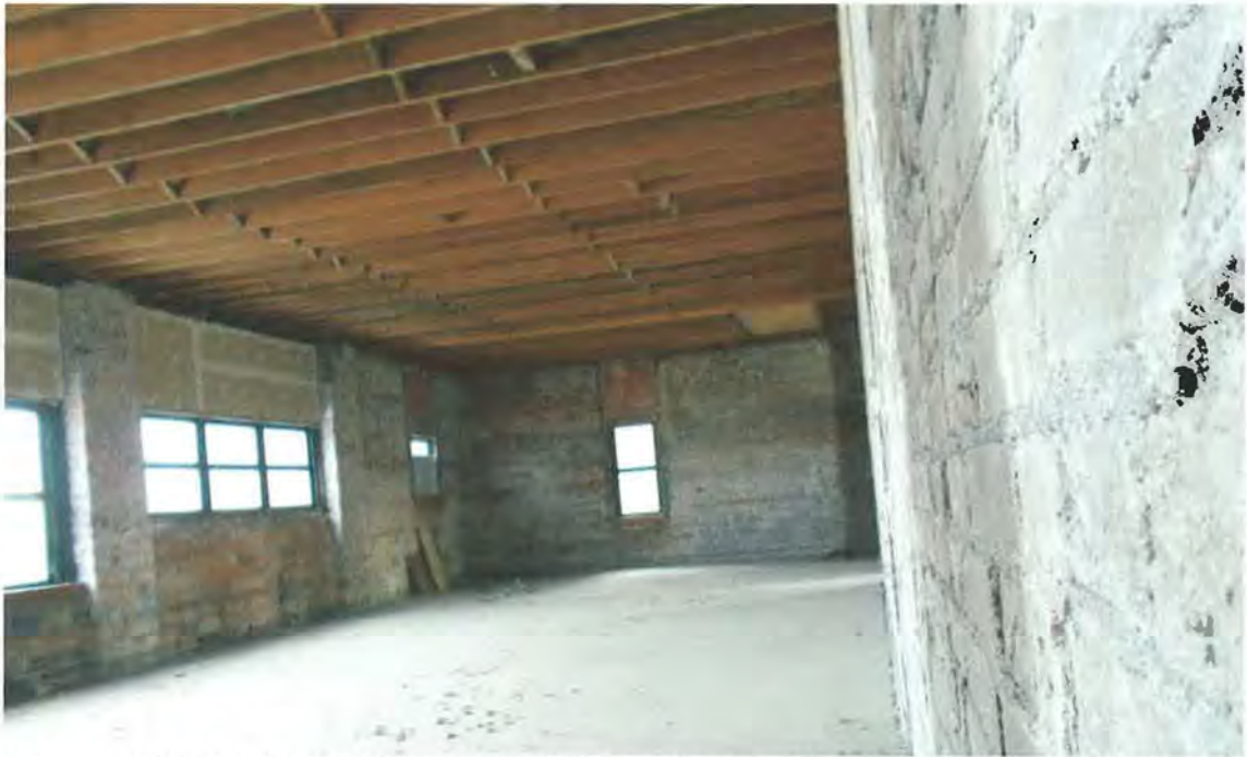
Third floor class room with both original and later room divider walls gone. The windows on the left overlook the alley and the lower roof of the foundry/forge/machine shop area. Tallgrass Historians L.C., 2015
