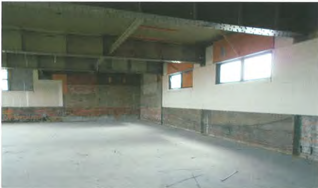
Gymnasium, 2 nd floor level. The concrete floor is newer and was installed after the perimeter running track at this level was removed. Note the plate girders at the ceiling and the pressed-metal ceiling cladding between the girders. Tallgrass Historians L.C., March 2015.
