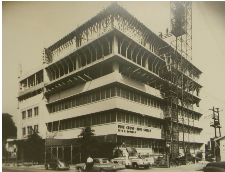
Beginning of construction of the upper floors circa 1968. (Photo courtesy of the Owner)
