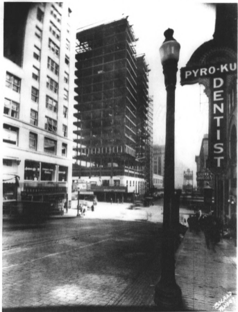
January 1, 1925. Washington Building under construction. West (main) and south facades, looking northeast. Tacoma Public Library. Marvin Boland photographer.
