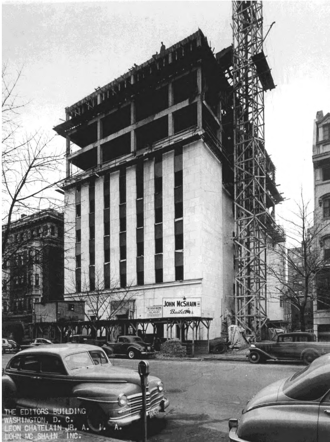
The Editors Building under construction, December 1949 (From personal collection of Leon Chatelain III, Chatelain Architects)
