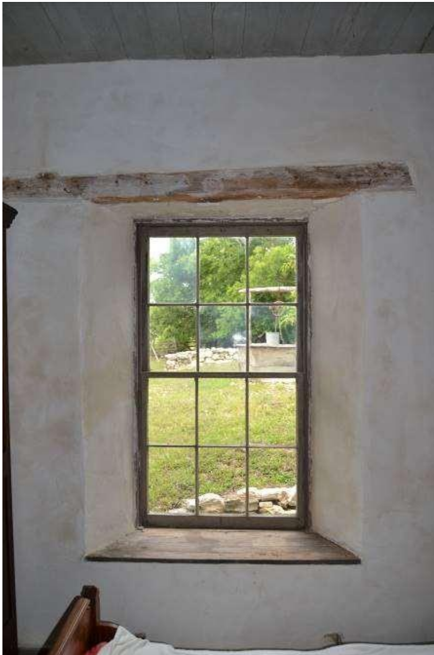
Photo No. 18. View of deep window sill in Room 5 (Resource A). View facing southwest.
