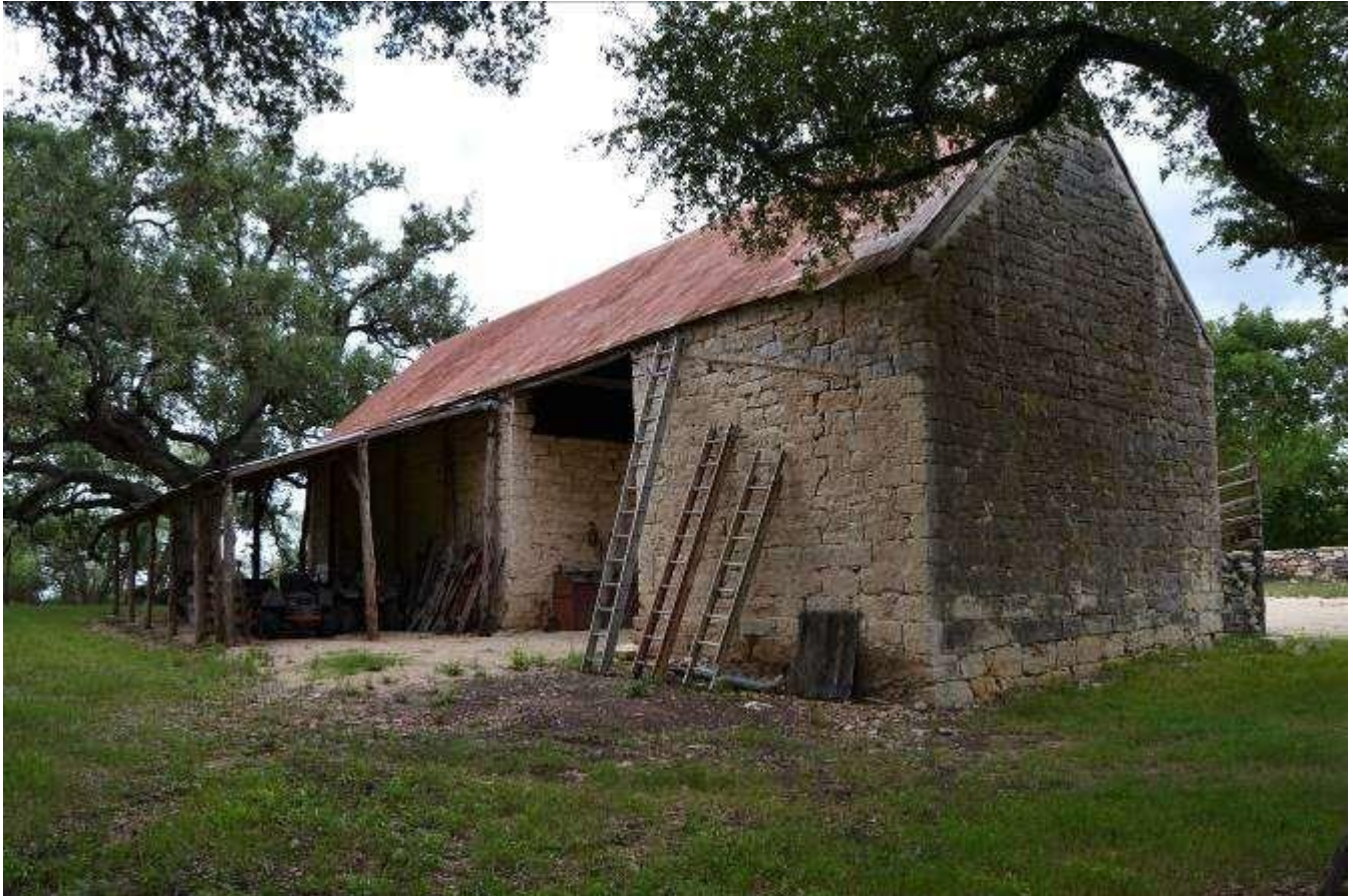
Photo No. 24. Oblique view of rear east and side north façades (Resource B). View facing south.
