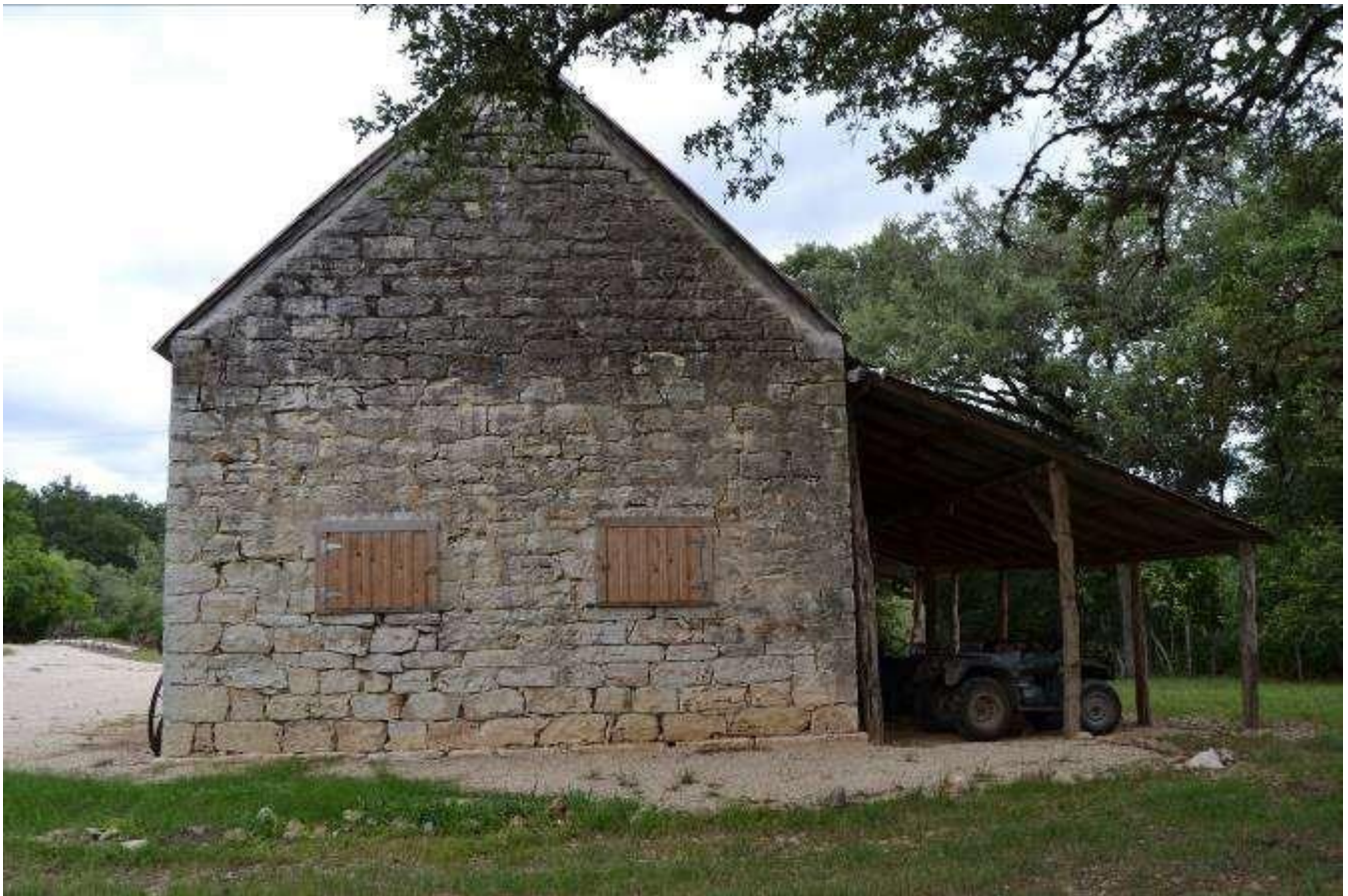
Photo No. 25. View of side south façade (Resource B). View facing north.
