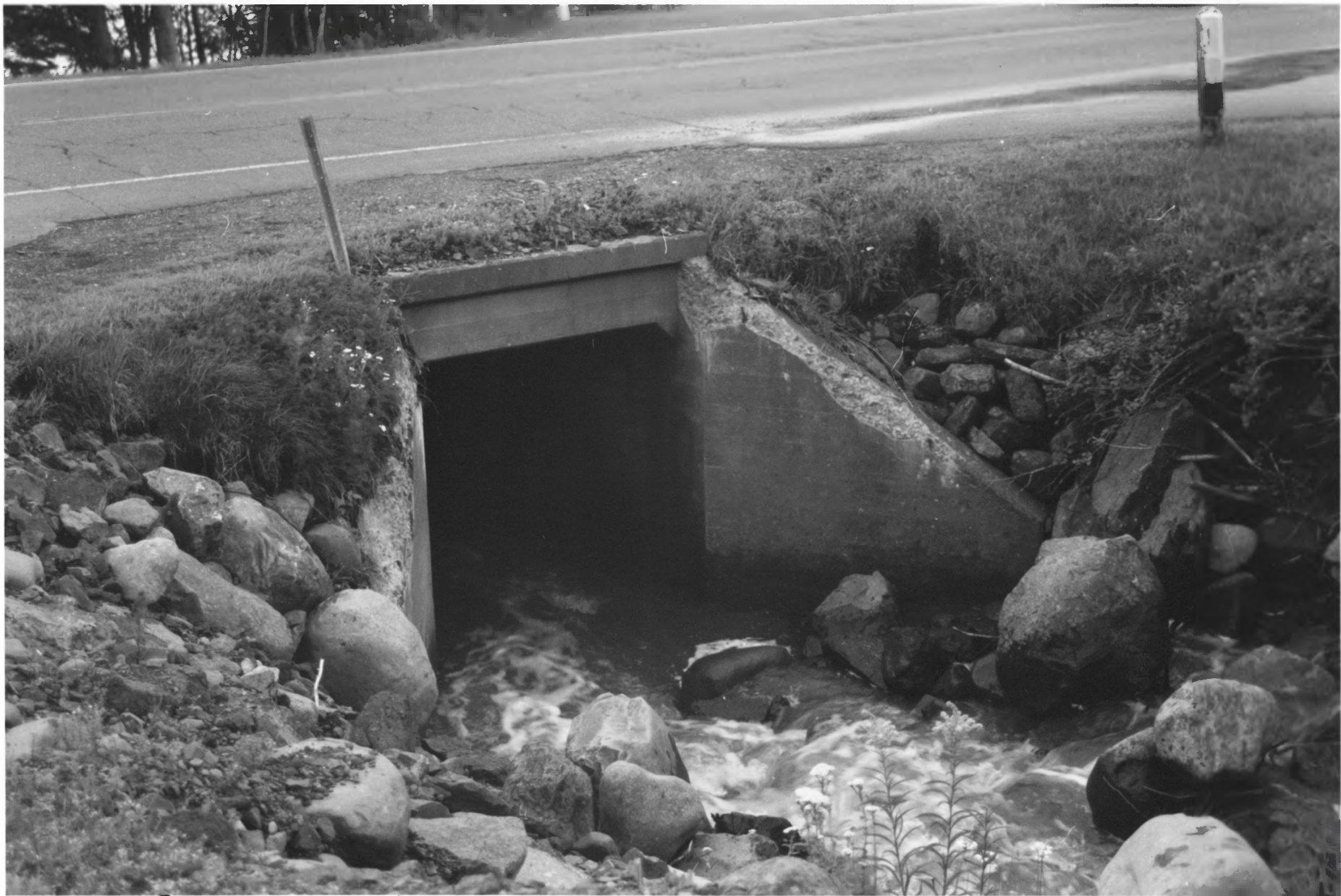
Cascade River Wayside Babineau Creek Culvert (NORTH SIDE) Cook Co., Mn 014535-10-B
