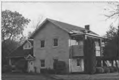
Cottage 7-9 is in poor condition on the interior and appears to have been altered substantially since their construction in the 1920s. Photos 2007 ARG.
