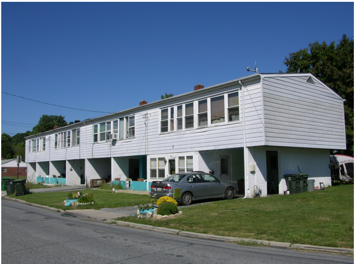
Photo 14: CC Plan 58-64 Foundry Street. One porch enclosed, all others and carports open. Camera facing W.
