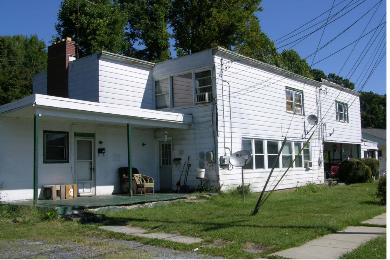
Photo 9: Plan A 4-plex (two units up and down). 61-67 Foundry Street. Addition to second level of East half. Camera facing NE.
